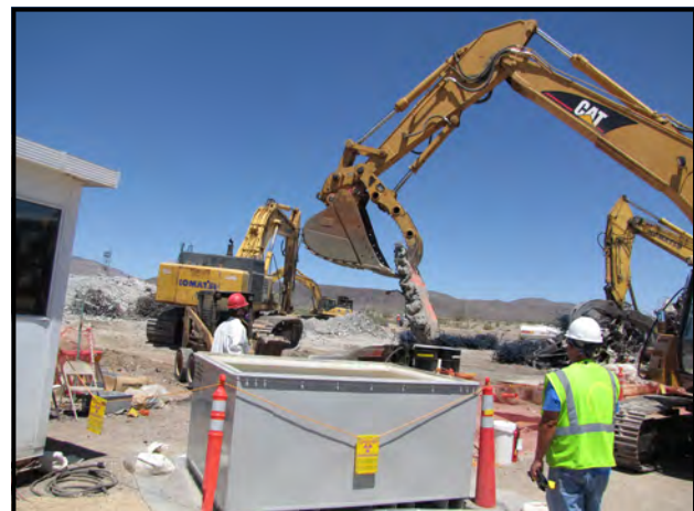
Workers remove mixed waste resulting from the demolition of the R-MAD facility at the Nevada Test.
