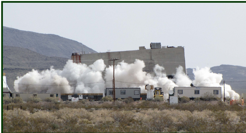
Crews perform demolition of the R-MAD facility. R-MAD is one of several Nevada Test Site facilities which supported the Nuclear Rocket Development Station program that ended in 1973.
