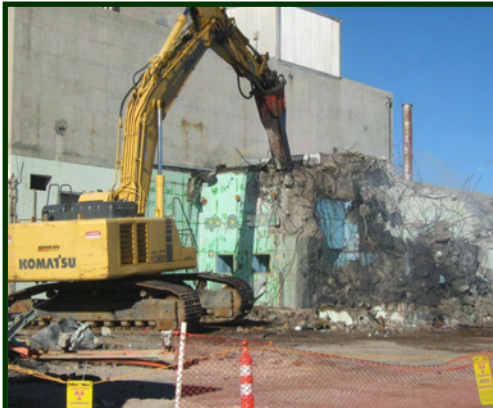
Phase I traditional demolition of R-MAD using a hydraulic hammer to dismantle a section of the south block wall and roof. A processor is used to size-reduce the resulting debris.
