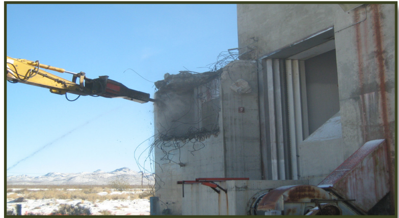
D&D activities at the Reactor Maintenance, Assembly, and Disassembly (R-MAD) facility using a hydraulic hammer.
