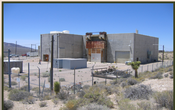
The Pluto facility was closed using the SAFER process. (before demolition, above, and during demolition, left)
