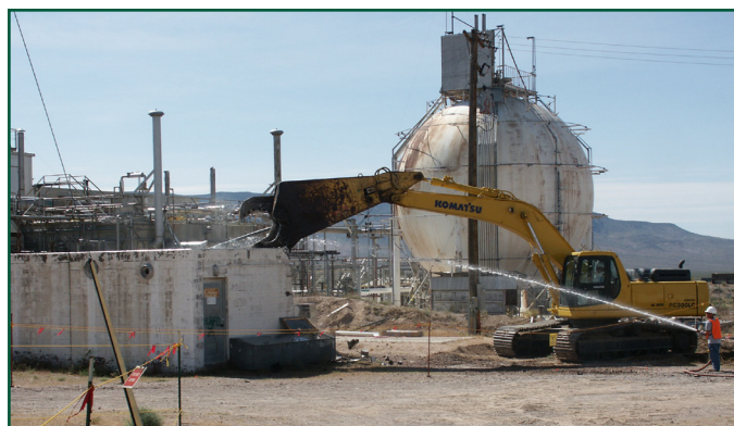
A worker sprays water for dust suppression as the hydraulic shears dismantle a building at the Test Cell A Facility on the Nevada National Security Site
