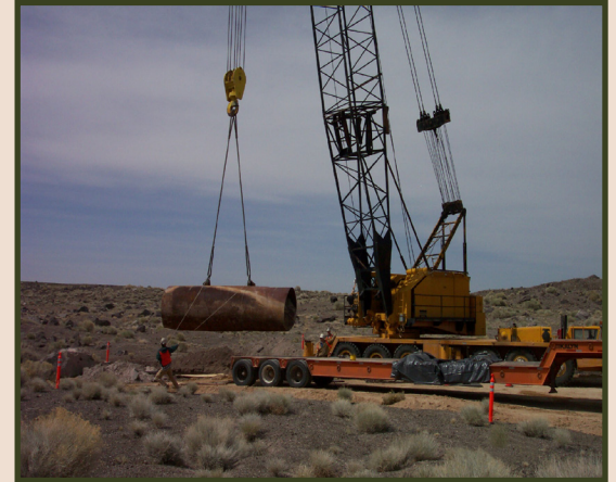
A crane removes an ordinary 6-by-20-foot steel pipe at a Housekeeping site on the Nevada National Security Site
