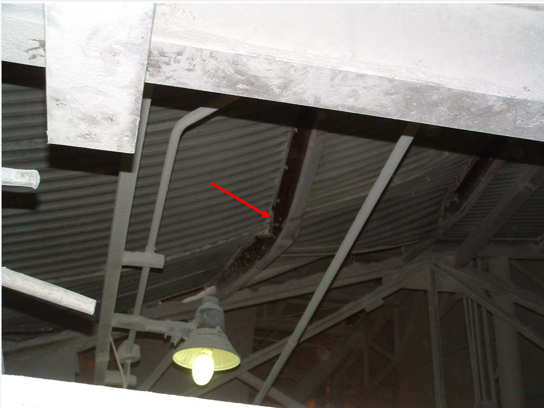
Collapsing Roof Support Purlins
