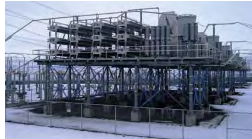
Series compensation devices, such as these at BPA's Schultz Substation, store voltage momentarily. Huge banks of them along lengthy transmission lines help keep the power system stable.
