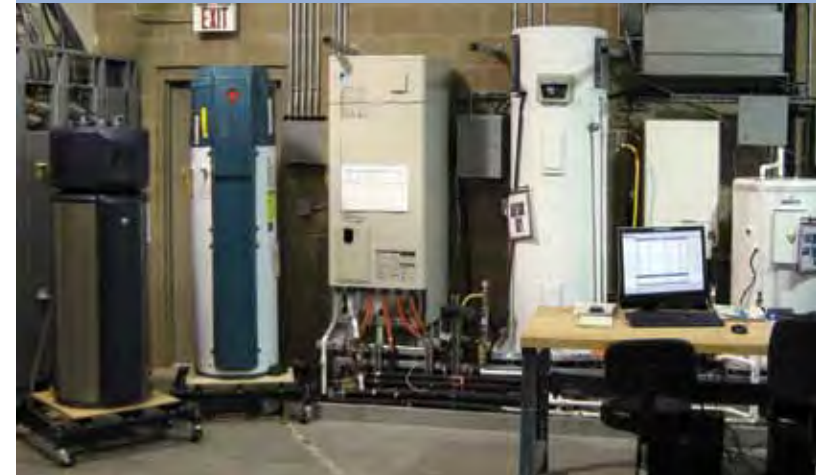
BPA and the Northwest Energy Efficiency Alliance are working to influence passage of federal standards requiring heat pump water heaters for all electric storage tanks. These heat pump water heaters are being bench tested in the Electric Power Research Institute’s Knoxville Living Laboratory.
