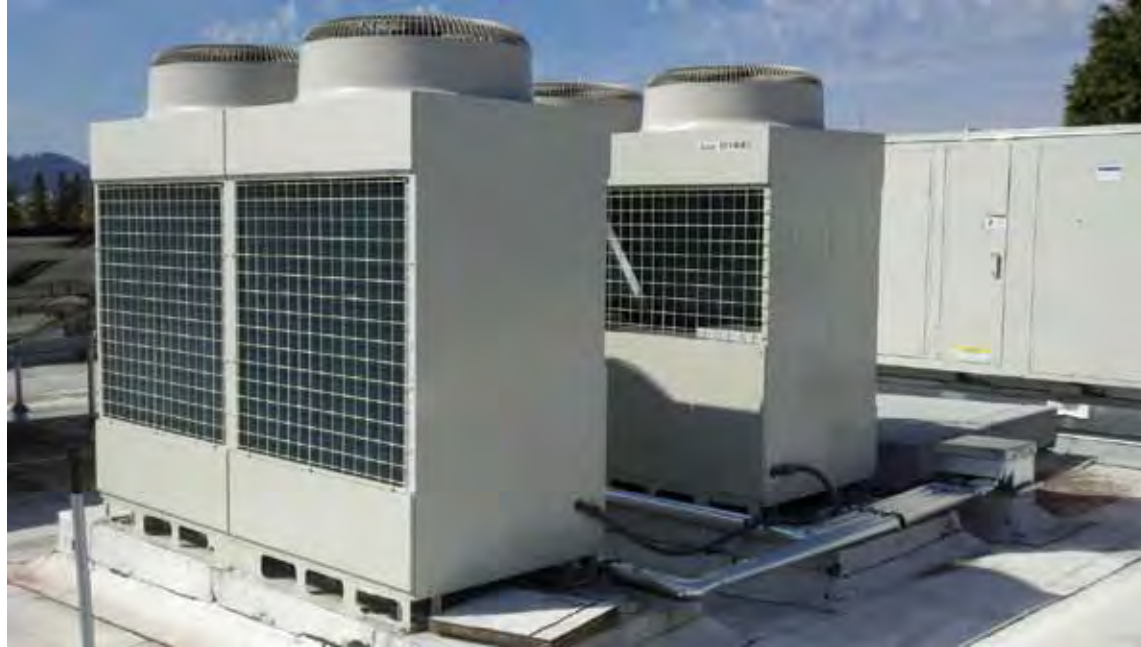
Roof unit, commercial building ductless heat pump.
