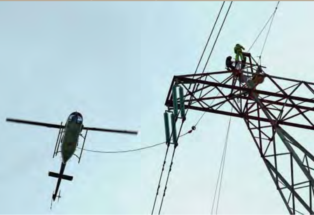
Using precision flying techniques, a BPA helicopter pilot helps crews string fiber optic cable.
