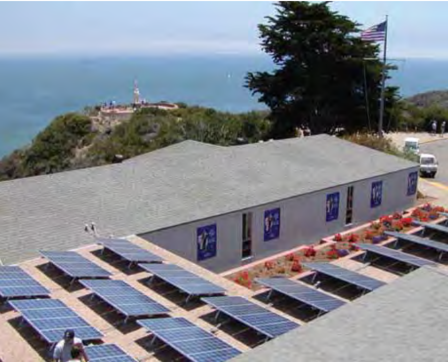
This 10-kilowatt photovoltaic array at Cabrillo National Monument in San Diego, was designed and contracted by BPA engineers under a reimburseable cost agreement with the National Park Service. Beginning in the mid-1990s, BPA contracted out to other public agencies to design and install energy efficiency and renewable energy system projects.
