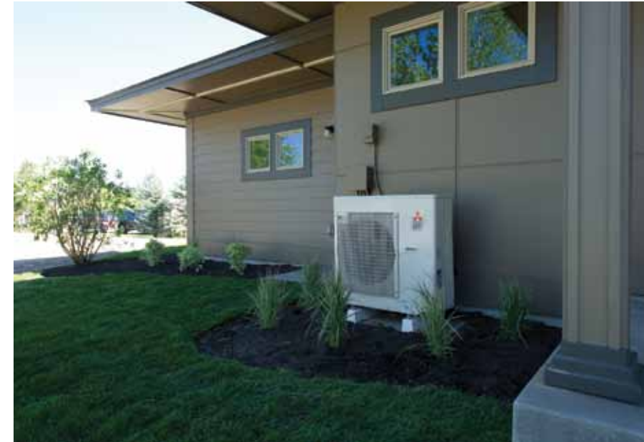
Ductless heat pumps (such as the outdoor compressor unit shown here) proved to offer significant energy savings for single-family homes when NEAA field tested them in 2006 to 2008. BPA was a major contributor to their success. In 2011, tests were under way to evaluate ductless heat pumps for use in manufactured homes, multifamily homes and small commercial buildings.
