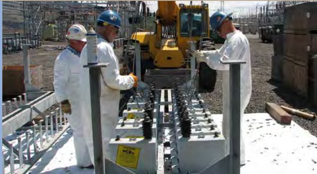
A rigging crew packages capacitors containing PCBs for disposal. The BPA crew, in blue hard hats, includes (from left) Walt Finney, Tom Wellman and (in the cab) Tom Thomas.
