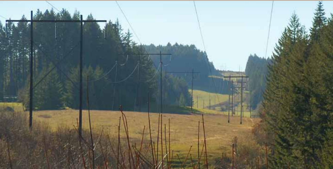
BPA replaced the wood poles on its Albany-Burnt Woods and Santiam-Toledo transmission lines in the summer of 2009. Vegetation stands well back from the lines.
