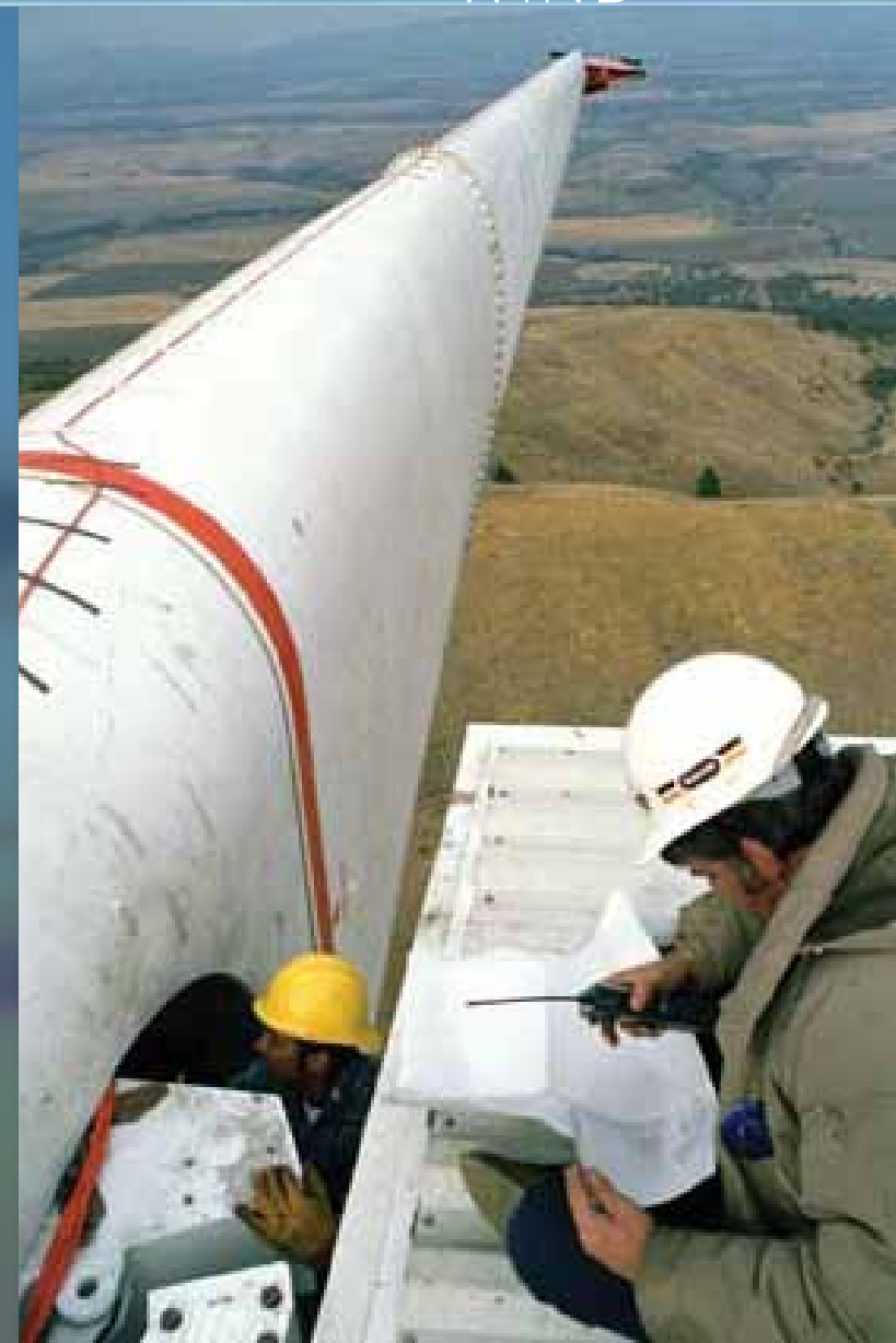
Technicians fine tune mechanisms inside a MOD-2 wind turbine. At 200 feet above ground, the generating units required a crane to move heavy pieces of equipment. (NASA)
