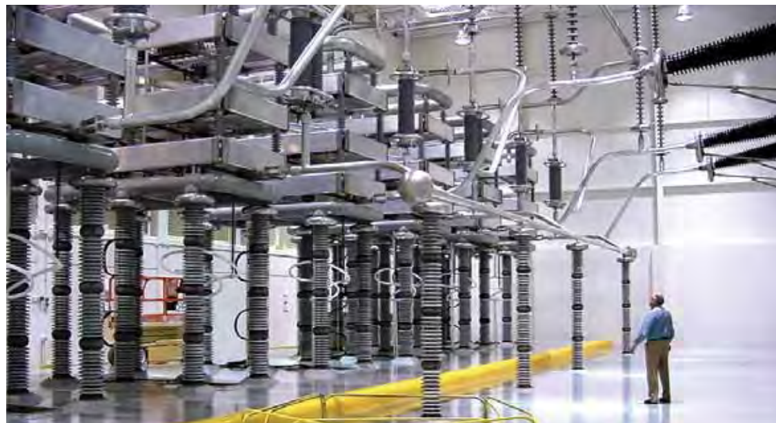
Modernization of BPA's Celilo Converter Station included replacement of decades-old mercury arc valves with solid-state technology to convert alternating-current electricity to direct-current for transmission to Southern California.
