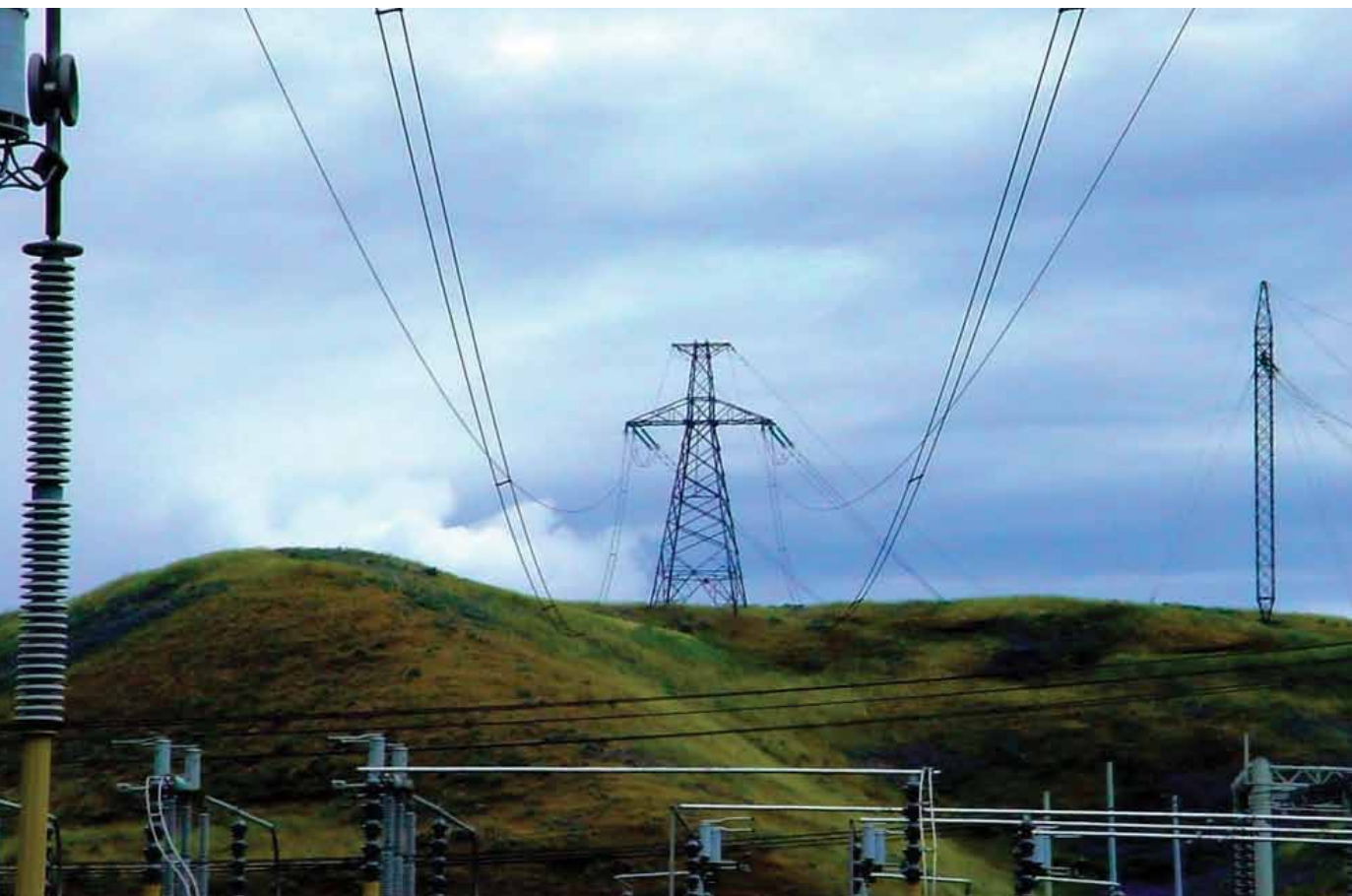
The direct-current transmission lines that begin the Pacific Northwest-Pacific Southwest Intertie stretch south from BPA's Celilo Converter Station in The Dalles.
