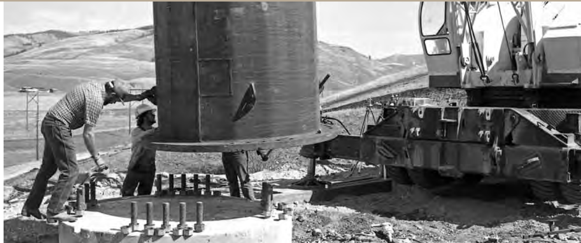
BPA included the public throughout the Colstrip project, including selection of the tower designs. The residents near one section of line selected single-pole towers, which BPA then designed and built specifically for this project.
