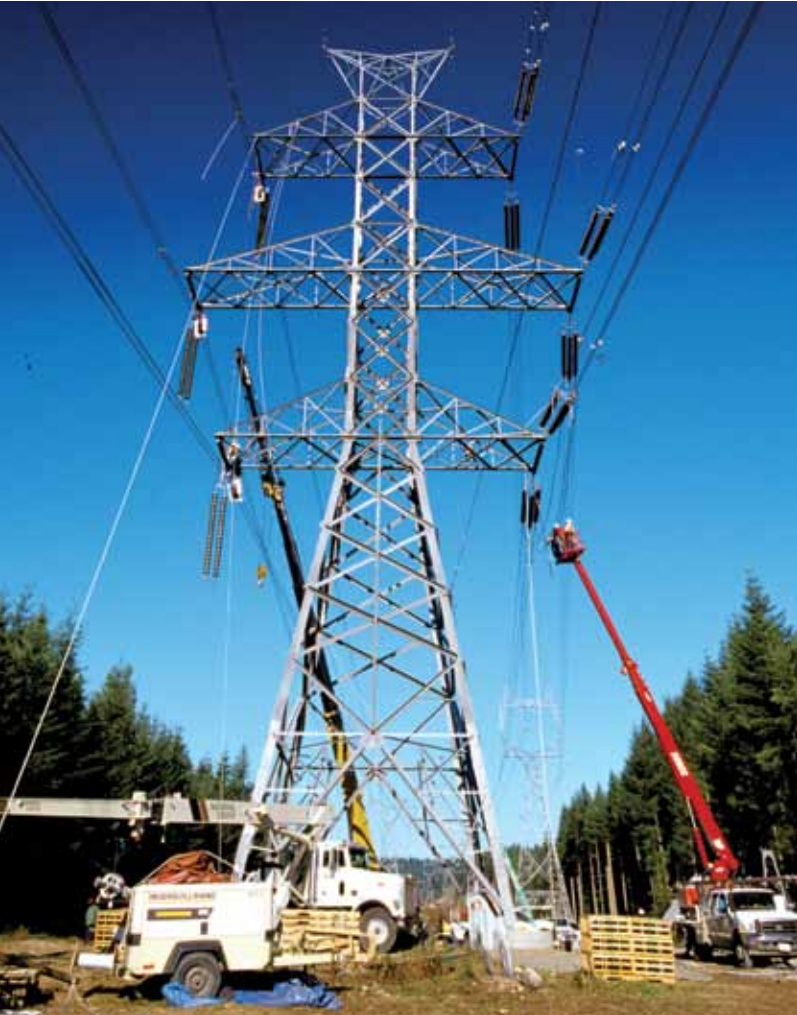
Double-circuit towers that support two sets of transmission lines helped reduce the environmental impacts of BPA's Kangley-Echo Lake line. (Lou Driessen/BPA)
