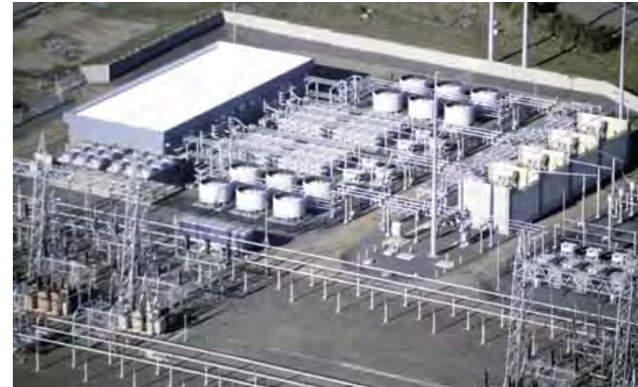
BPA's Keeler Substation (below), near Portland, is home to the fast-acting devices (above) which help stabilize power swings on the system caused by short circuits or other disturbances.
