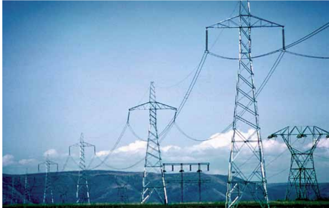
Improvements doubled the capacity of the direct-current intertie, in the foreground, without adding to the wires already in the air.
