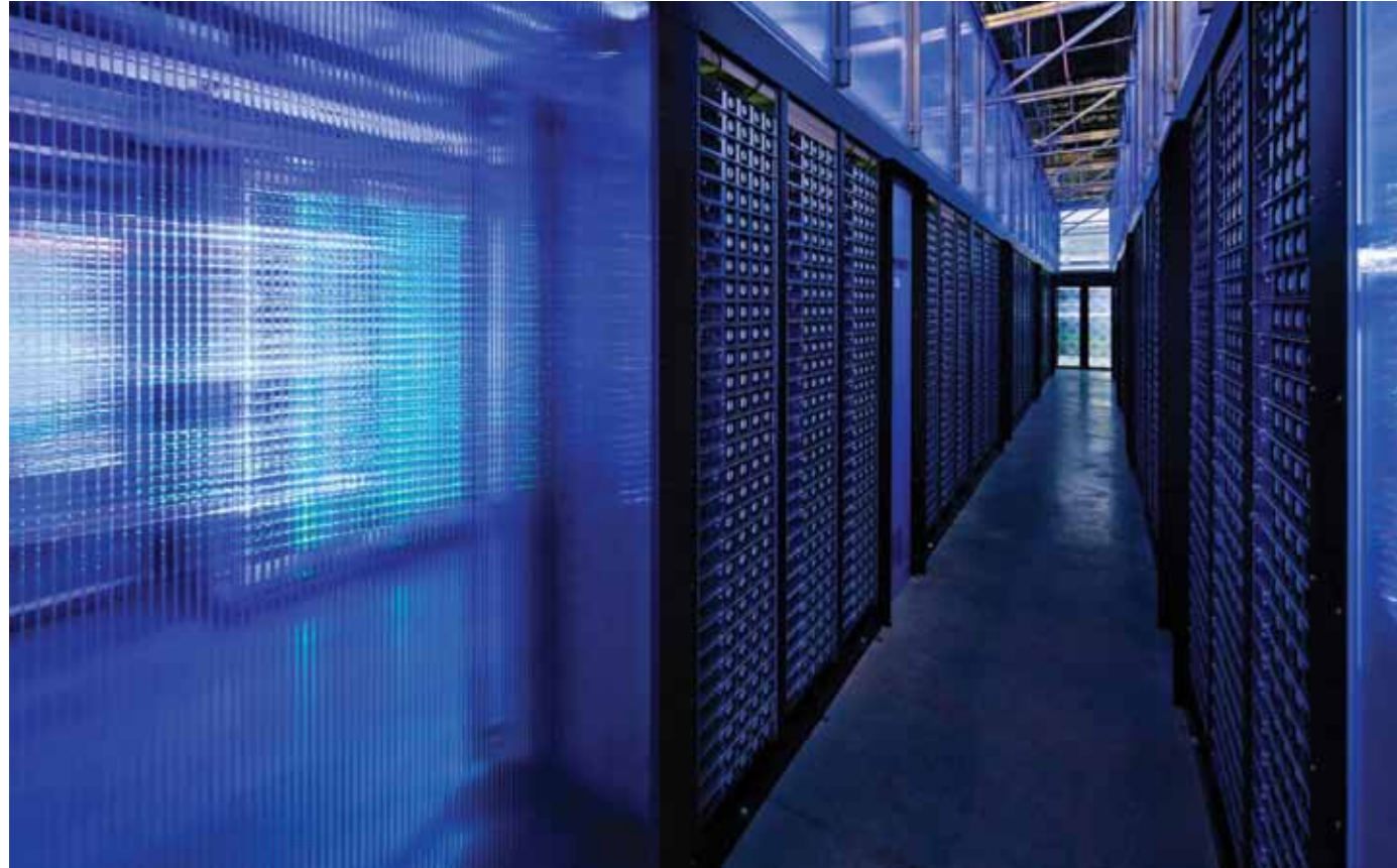
The efficient design of Facebook’s data center in Prineville, Ore., reduces energy consumption. BPA’s transmission system helps supply the data center with electricity. (Facebook)
