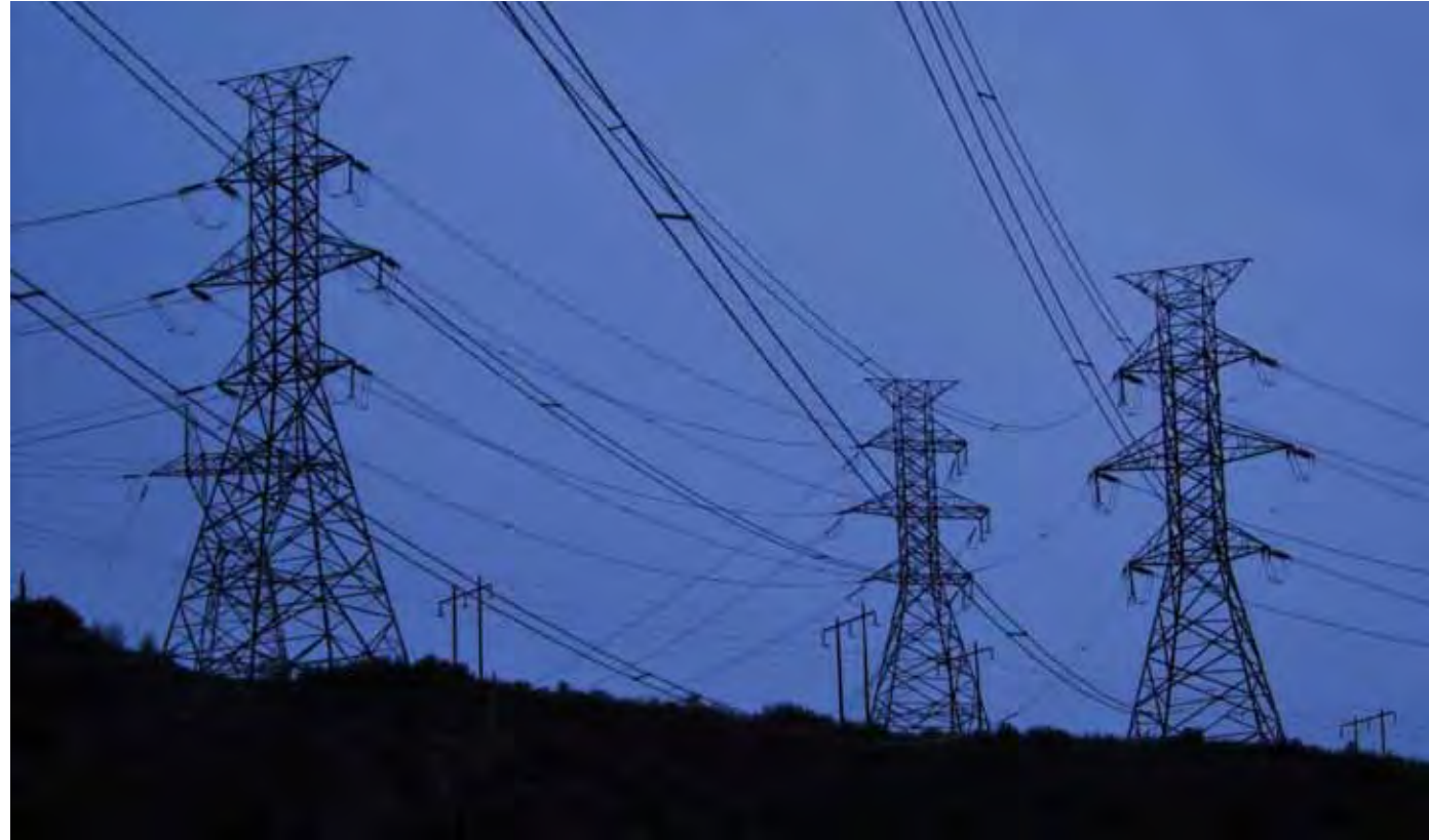
BPA transmission lines carry power from Grand Coulee Dam, one of the largest power plants in the nation, throughout the Northwest and beyond. (David McNew/Getty Images)
