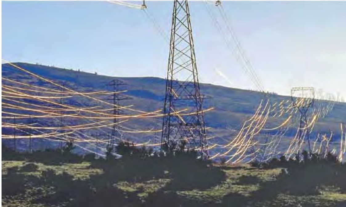
Transmission lines connected to BPA's Schultz Substation near Ellensburg, Wash., helped BPA avoid stretching a new line across the Cascades.
