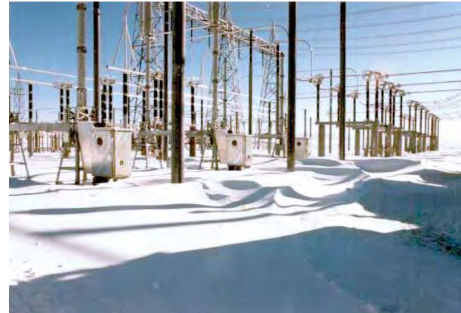
During a Montana cold snap in 1989, equipment at Garrison Substation choked in the sub-zero temperatures.
