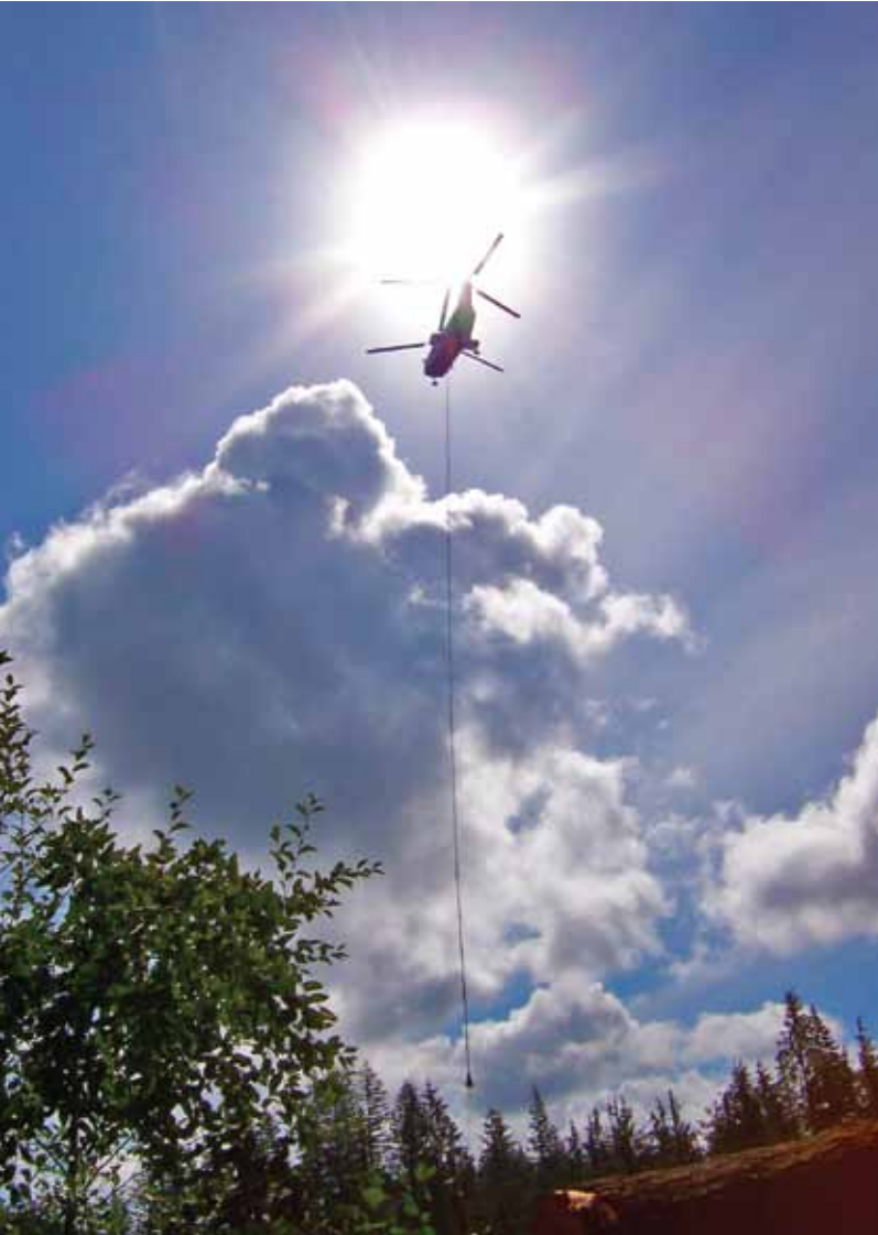
A helicopter lifts tower sections into place on the Kangley-Echo Lake line to minimize impacts on the ground.
