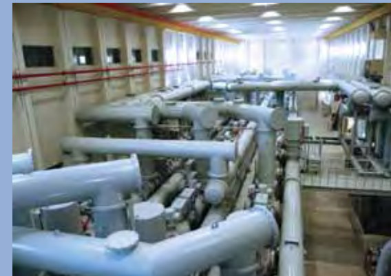
Squeezing a 15-acre substation into a 60-by-200-foot building keeps Taft Substation operating despite snow that can be 10 feet deep in a typical winter.
