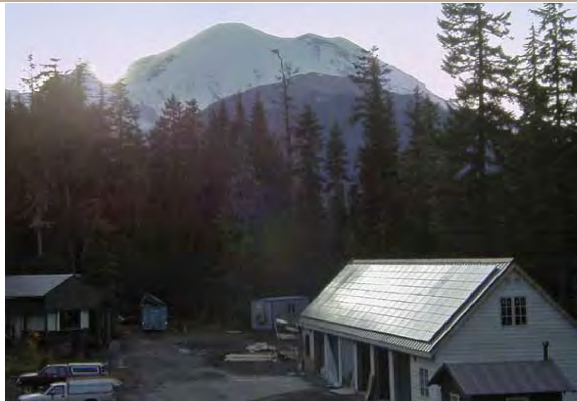
This 20-kilowatt photovoltaic installation was contracted by BPA engineers on a service building at Mt. Rainier National Park; it operates off the transmission grid, dramatically reducing the use of a diesel generator.
