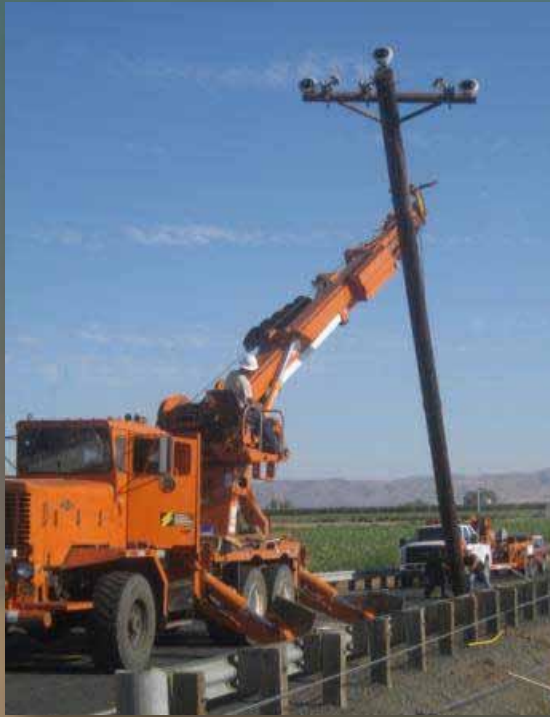
An all Native American line crew from Yakama Power replaces a damaged power line in June 2011 with a truck on loan from BPA. The Yakama Nation formed its own utility, with assistance from BPA, and began purchasing power to serve members near Toppenish, Wash., in 2009. (Yakama Power)
