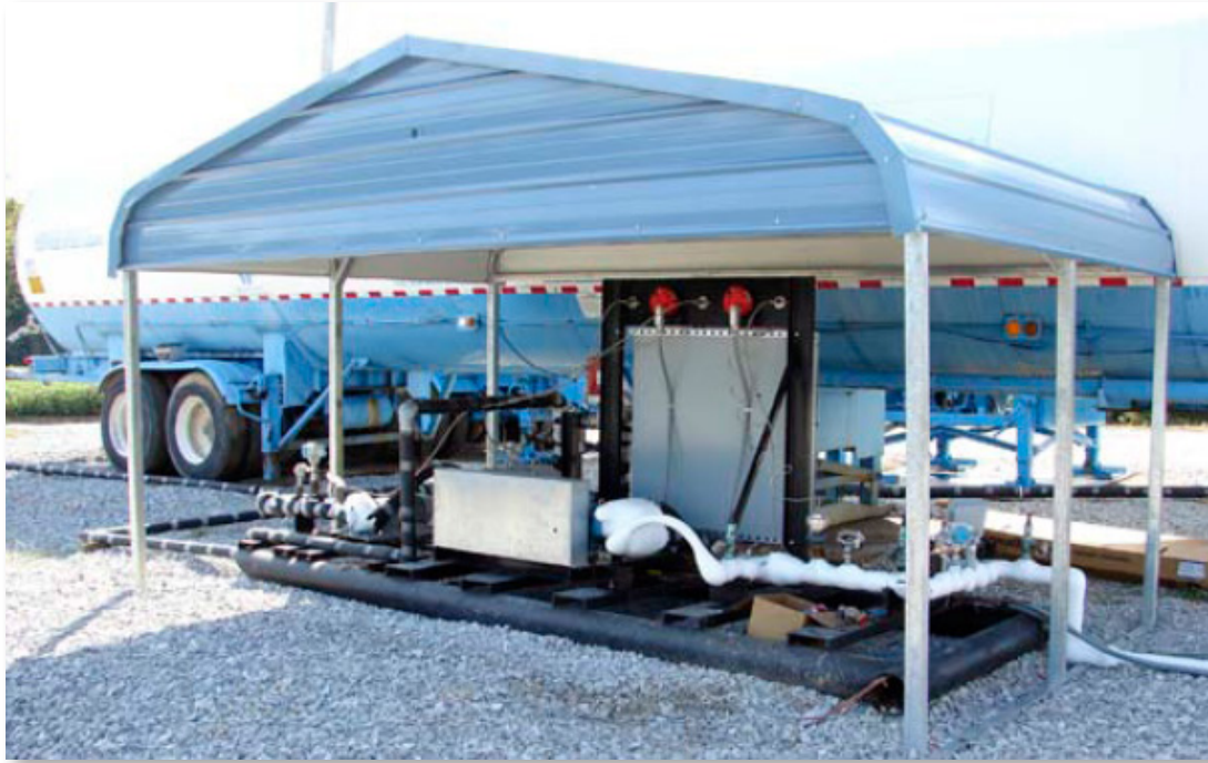
Injection pump skid with CO 2 supply tanker in the background, Mumford Hills Test site
