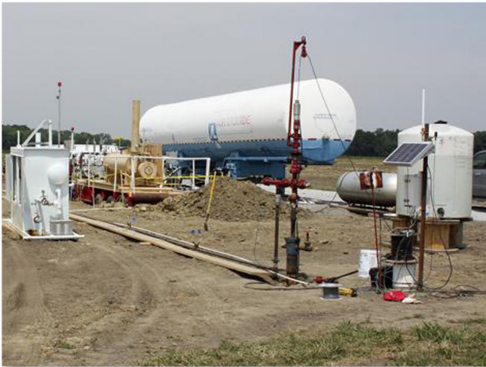
Injection Equipment and Wellhead for MGSC CoalTest
