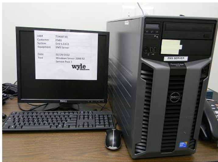
Photograph No. 10: EMS Server
