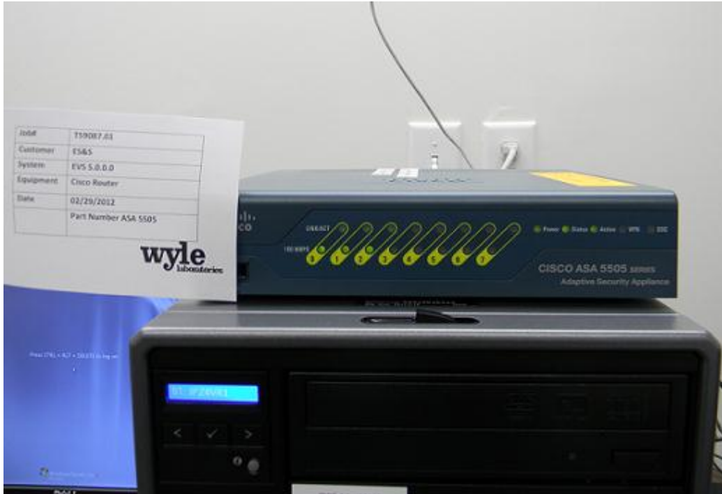
Photograph No. 8: Cisco Router Front View
