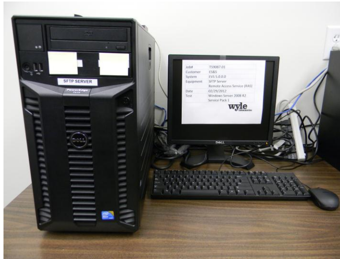
Photograph No. 9: SFTP Server Configuration
