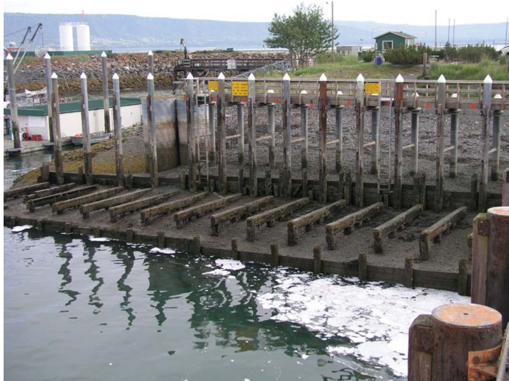
Figure 50. Grids used for boat hull cleaning and maintenance operations in Homer Harbor.
