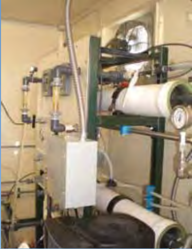
B.E.S.T. water cleaning equipment.
