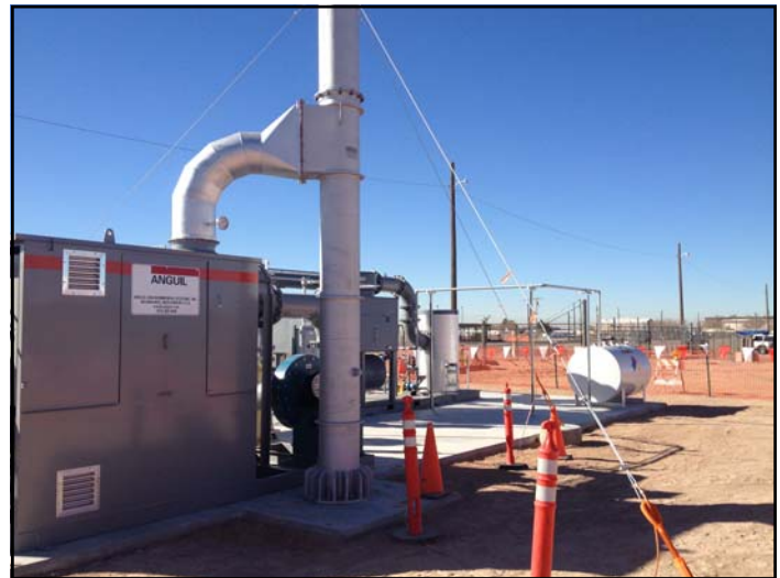
New soil vapor extraction unit at Kirtland Air Force Base
