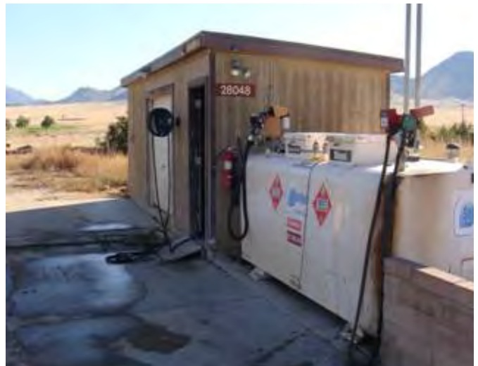
Wash rack is a recurring source of water quality concerns.
