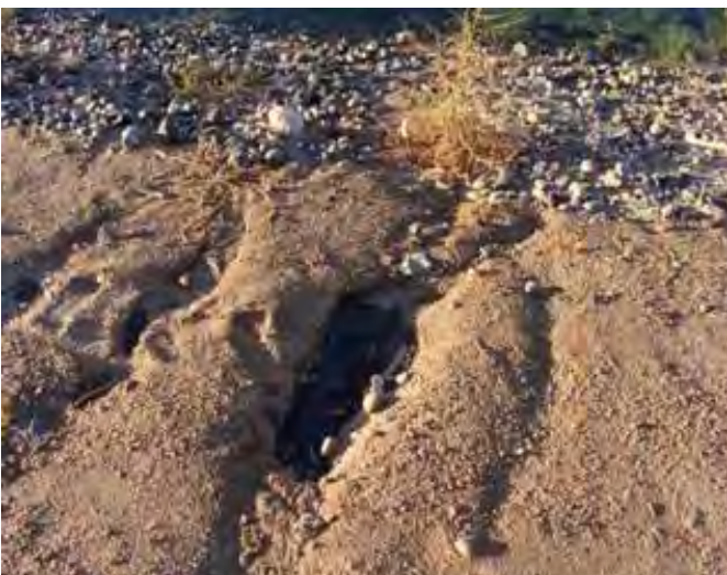
Soils are eroding into the golf hazards/Well#7 ponds.
