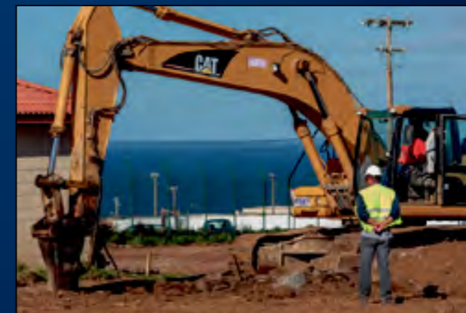
The construction site supervisor watches while the grounds are prepared for a new septic system during renovations at the old American Forces Network building, Nov. 8, 2012, Lajes Field. (Photo by Lucas Silva)
