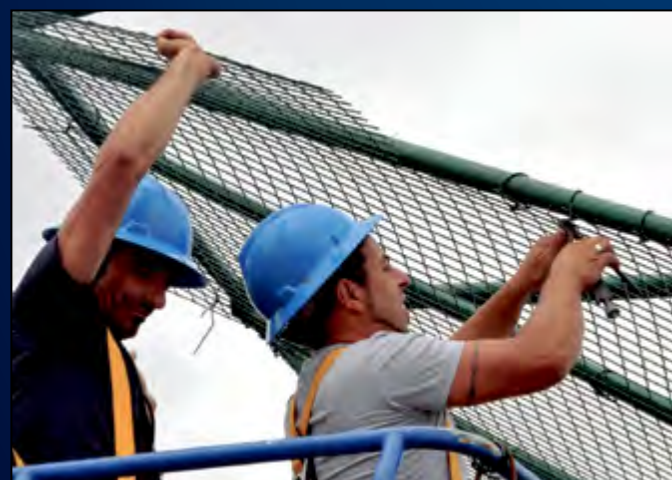
Paulo Inacio and Marco Machado install in a new fence at the softball field Aug. 28. More than 700 local national employees help Team Lajes complete its mission. (Photo by Guido Melo)
