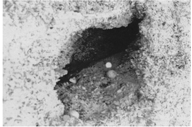
Figure 4-7. Piping and seepage in bank
