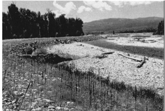
Figure 3-8. Bank protection necessitated by encroachment on levee setback
