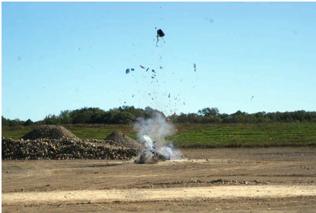
Figure III-6. Bomb blast site in an old landfill in Williamsport, PA.
