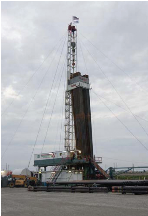
Figure 21. MGSC Phase III Injection Well. (Courtesy of MGSC Website)
