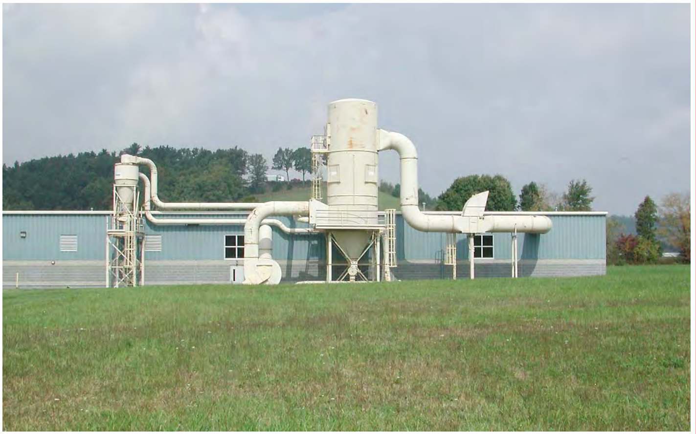
DUST COLLECTION SYSTEM
