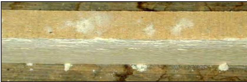
Figure 12-3. This severely infested drying stick also shows damage ranging from bore holes through the surface of the wood to frass accumulation. Note: Drying sticks should be heated to at least 130°F to destroy infestations and prevent insects from spreading to valuable lumber.
