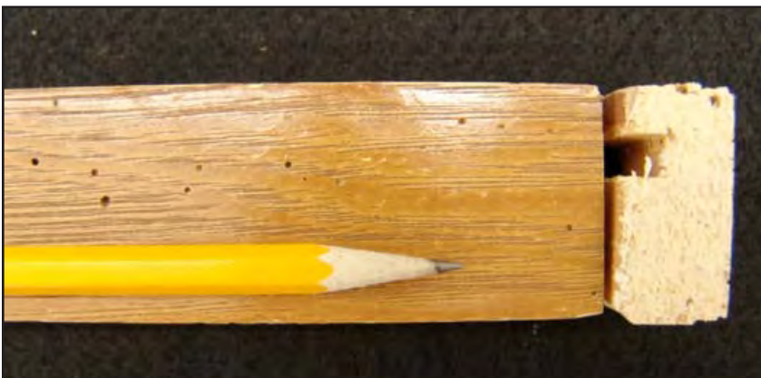
Figure 12-4. Powderpost beetle damage can also occur after a product is manufactured from infested wood and installed, as in this cabinet rail. At this point, the wood product has to be removed or treated in place. Once the wood is finished, the insects are not likely to penetrate the smooth surface and reinfest it.
