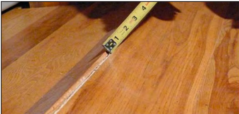
Figure 11-8. The hardwood floor buckled due to moisture regain during winter months.
