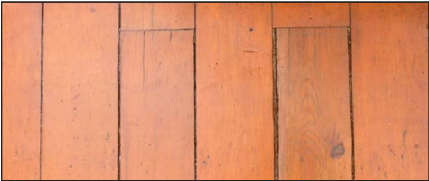
Figure 11-7. Wide cracks between 130-year-old white pine floor boards.
