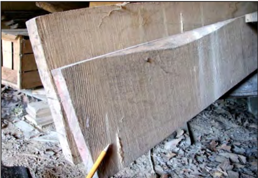
Figure 12-2. Wood boring beetle damage is usually detected when piles of frass or powder accumulate under the insect exit holes. The powder may also stream down the side of the infested lumber, such as on these old hard maple boards stored in a barn.
