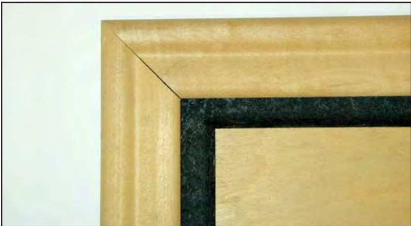
Figure 11-2. The miter joint has opened up on the inside due to shrinkage.
