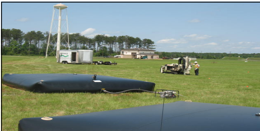
Emulsified vegetable oil and bioaugmentation culture are injected into the substrate to treat the TCE plume at the Former Weapons Maintenance Area (SS-32).
