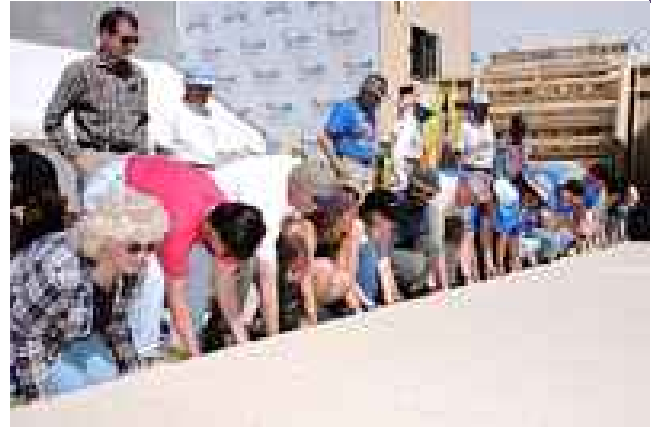
Sandia volunteers prepare to hoist a wall section into place as they begin the Rodriguez family house.
