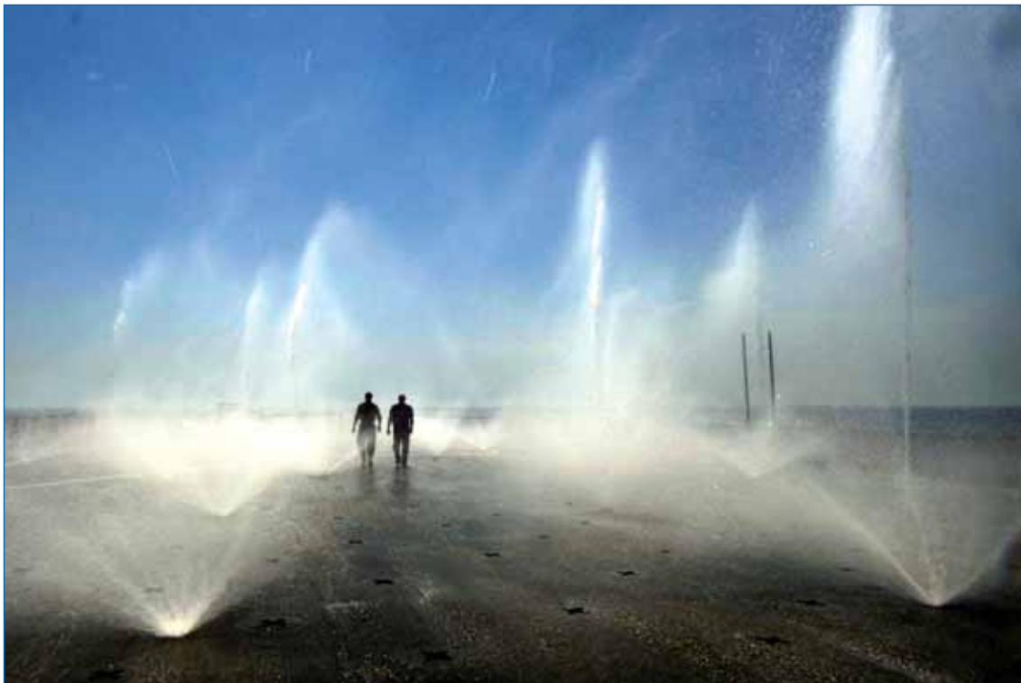
Sailors assigned to USS Ashland (LSD 48) inspect the sprinklers and valves of the chemical, biological, and radiological wash down system on the ship's flight deck.
