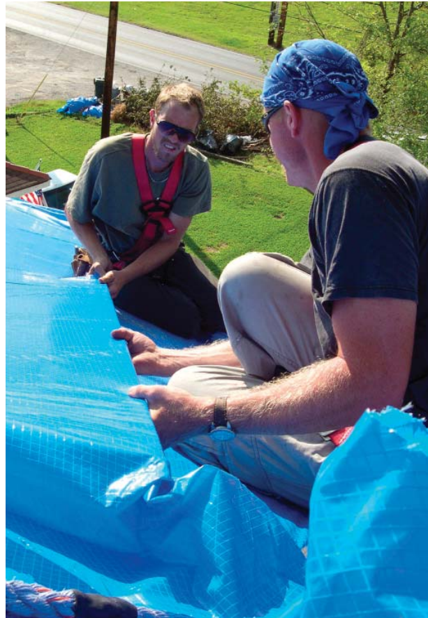
Corps of Engineers contractors install a blue roof on a house in eastern Jefferson Parish, Louisiana in support of Hurricane Katrina recovery efforts.
