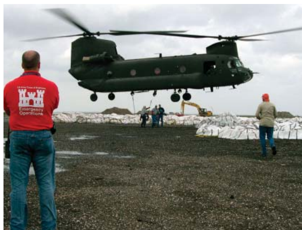
U.S. Army Corps of Engineers New Orleans District Project Manager Stuart Waits watches as workers hook up cables to an Army National Guard CH-47 Chinook helicopter to lift 5,000 pound sandbags for transport to the Industrial Canal in New Orleans.
