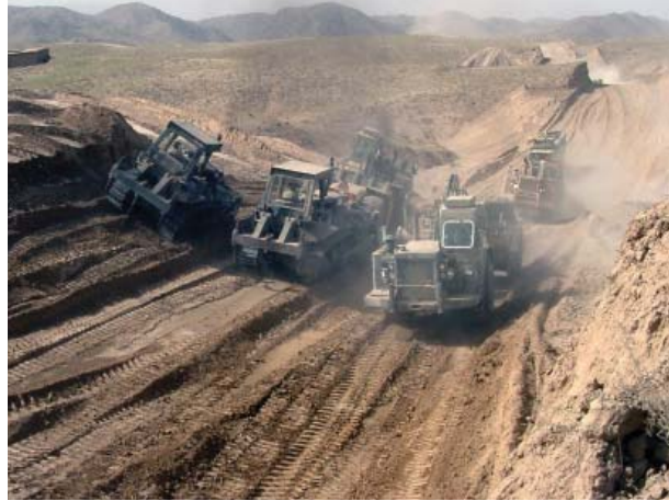
Army engineers from Alaska-based Company C, 864th Engineer Combat Battalion, level a portion of the nearly completed 117-kilometer TK Road, stretching from Kandahar to Tarin Kowt, Afghanistan. (by 1st Lt. Laura Walker)
