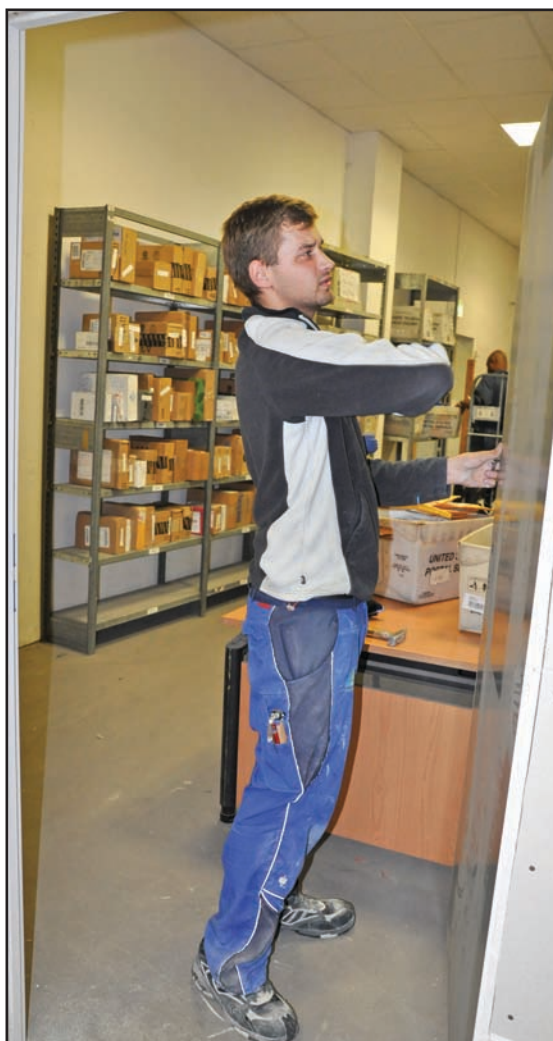
Kevin Block works on installing a new wall and doorway to serve patrons at the parcel pickup area in Wiesbaden's Postal Service Center.
