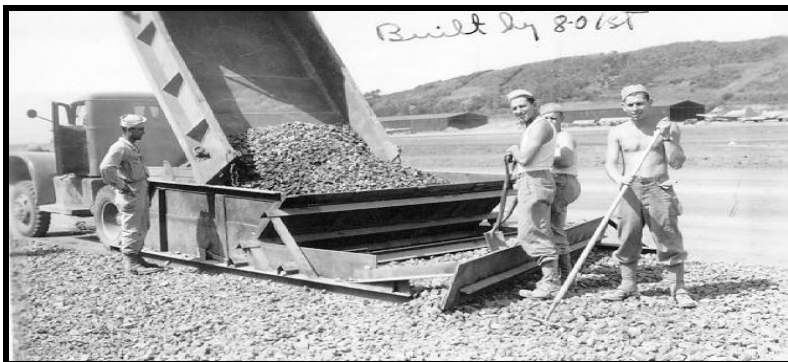
Engineers from the U.S. Army 801 st Engineer Battalion constructed a runway at Lajes in 1944.
