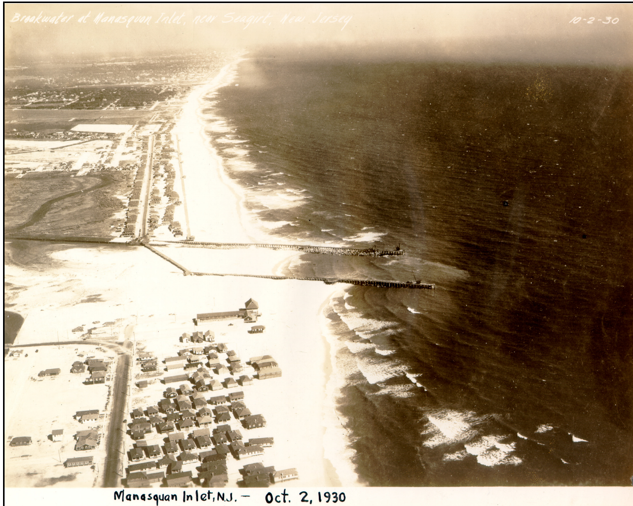
Figure I-3-9. Construction of Manasquan Inlet jetties, New Jersey, October 2, 1930, view looking north. Material for the jetties was supplied via an elevated roadway that extended out to sea from the land. Note that sand is already accumulating on the south (lower) side of the south jetty. The shoreline is continuous, and at this site the inlet was dredged after the jetties were completed. Other man-made openings that are now Federal navigation projects include Panama City Inlet, Florida, Duluth Cut, Minnesota, and Aransas Pass, Texas. (Photograph from Beach Erosion Board archives)
