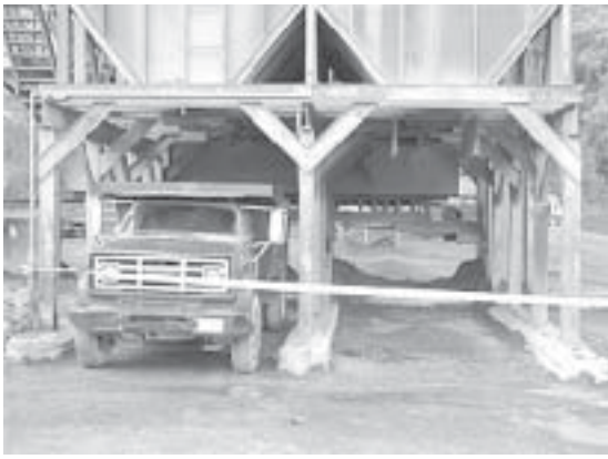
Photo of the side-by-side load-out bins.
