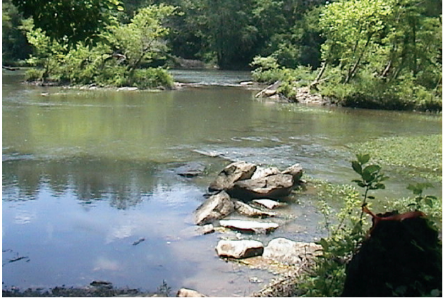
Stream crossing undergoing repair, Big South Fork National River and Recreation Area (Bakaletz, 2006).
