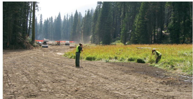
Grades were checked constantly during construction to make sure that cross-sections were flat (Wagner, 2007).
