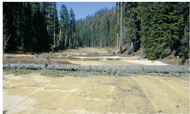
Once construction was finished, water was released into the upper meadow and is spreading and sheetflowing as designed (Wagner, 2007).
