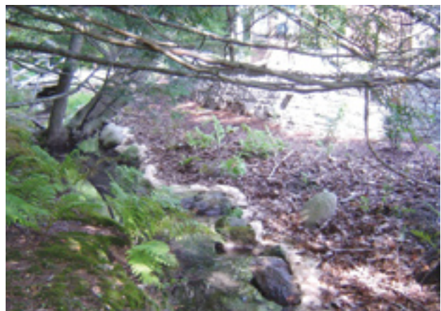
Acadia National Park staff completed a streambank stabilization at Sieur du Mont (Ellsworth, 2006).
