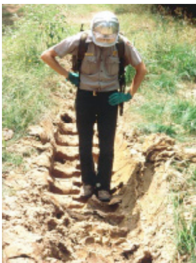
Ditching through park wetlands is a primary concern when dealing with oil and gas production (NPS, 2006).
