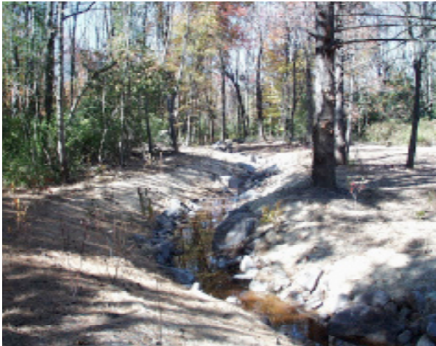
A portion of the daylighted stream after grading and planting (C. Davis, 2006).
