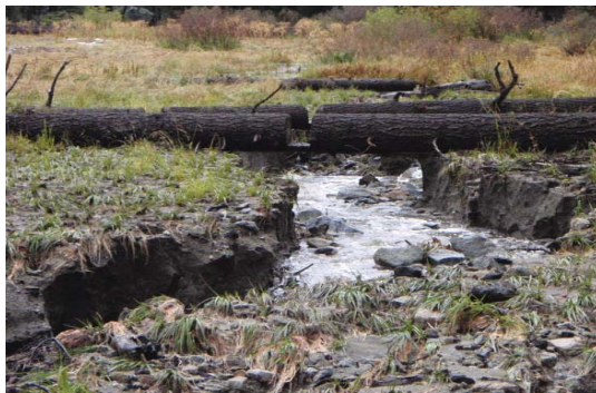
Storm damage in the meadow (eroded channel)
