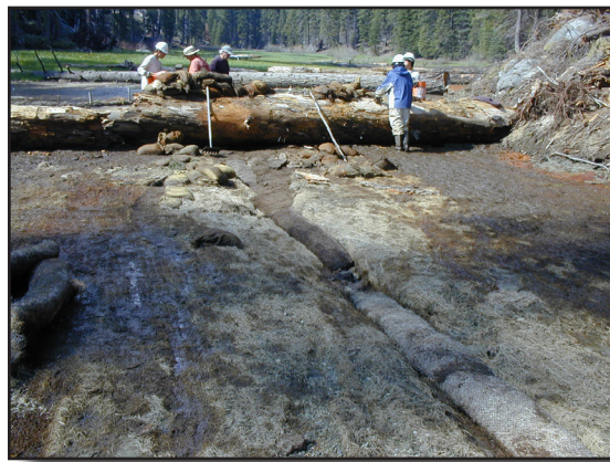
Filling minor erosion channels with coconut fiber logs and dirt, Upper Halstead Meadow, Sequoia National Park (Demetry, May 2008). Large logs were placed in 2007 to slow water flow.
