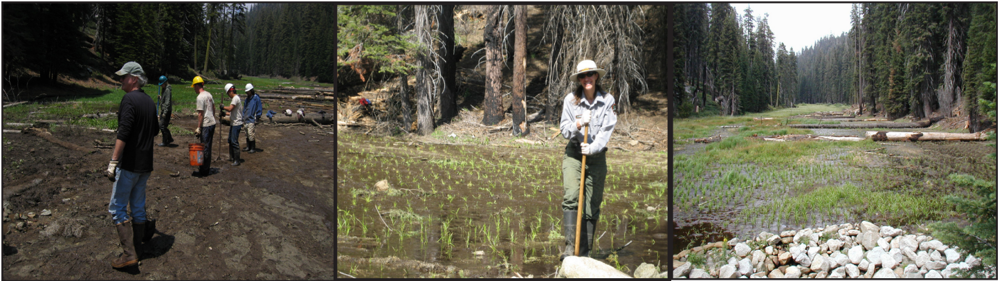
WRD staff and volunteers treating minor erosion channels at Upper Halstead Meadow after a wet winter, Sequoia National Park (Wolf, May 2008).
