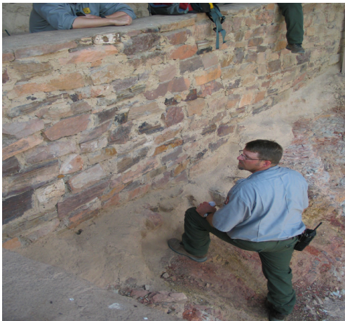
Examining ruins for water damage at Tonto National Monument (Reber, 2008).
