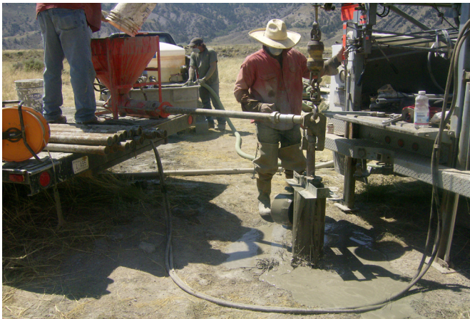
Closure of thermal well near Mammoth, WY in Yellowstone National Park by pressure grouting (NPS 2008).
