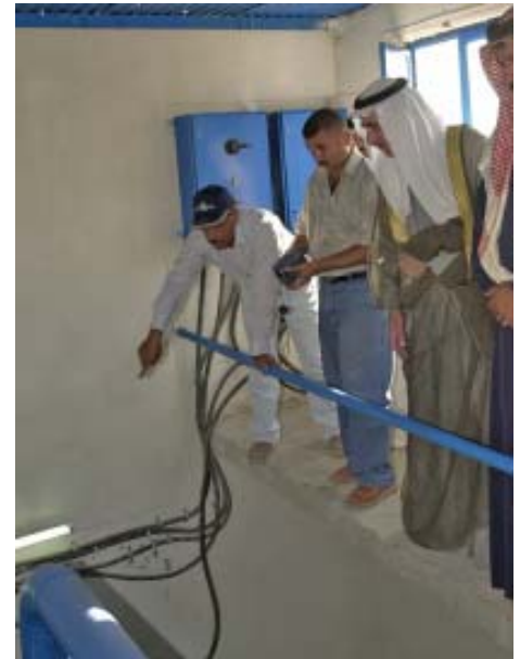
Mandu Hazali, project coordinator, shows new pumps to Owja city council members Sept. 7.
