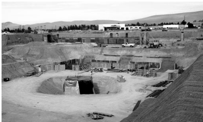
FIGURE 15. Excavation and forms for the NIF target area at year's end. (40-60-1197-2342#1pb01).
