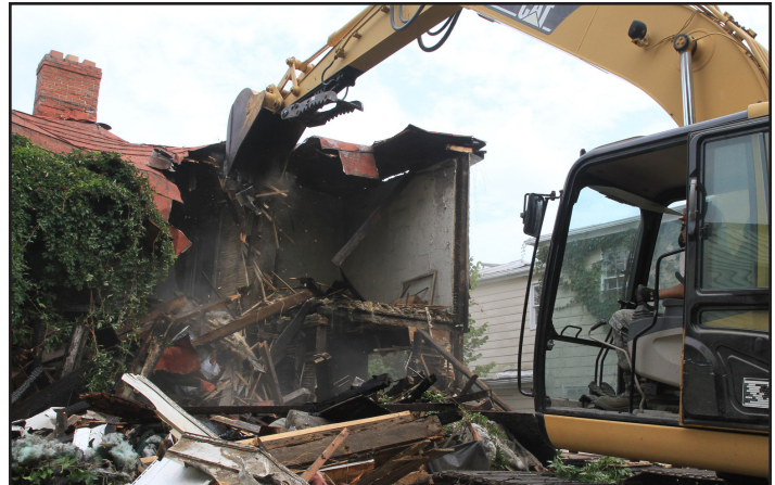
Airmen from the Virginia Beach-based 203rd RED HORSE Squadron use heavy equipment to demolish derelict structures associated with the drug trade Aug. 22 in Petersburg.
