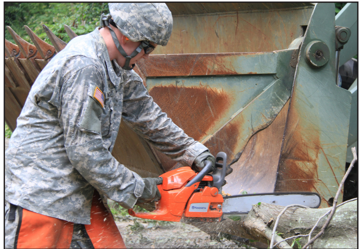
Soldiers from the Virginia National Guard's Cedar Bluff-based 1033rd Engineer Support Company, 276th Engineer Battalion, 91st Troop Command work to clear a path for the Cannon Creek pedestrian and bike trail July 17 in Richmond.
