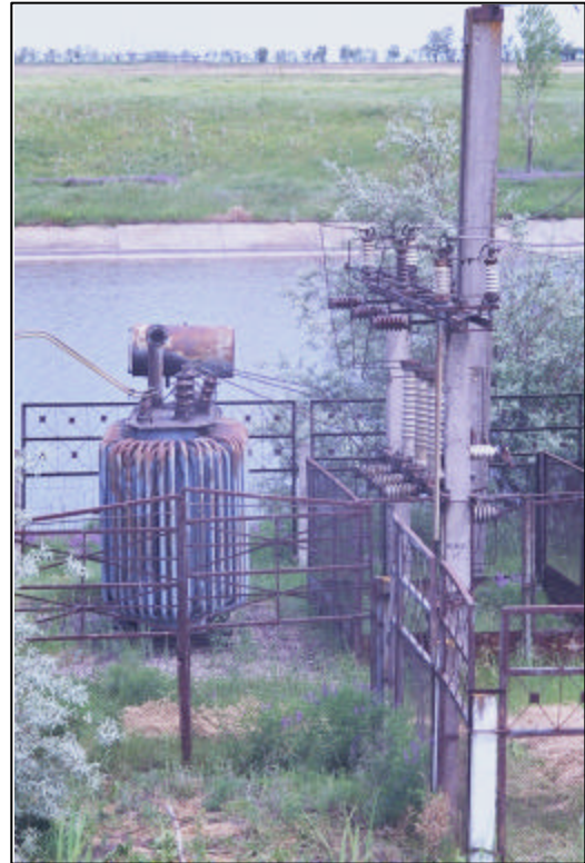
Transformers using PCBs are common along irrigation canals, where leakage is a threat to local terrestrial biodiversity and aquatic biodiversity far downstream. Photo by D. Gibson.
