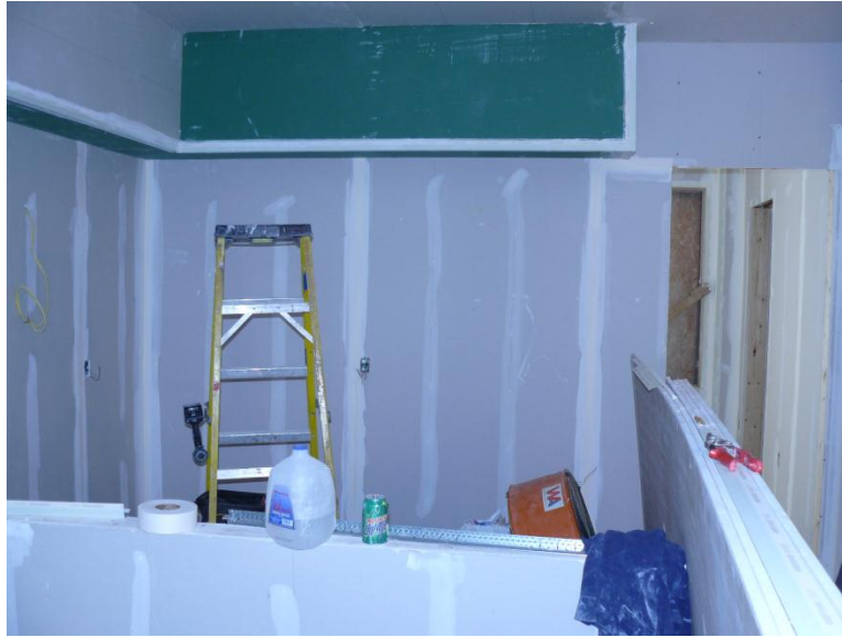
Interior photo of an upper level apartment unit for which the work was not complete
