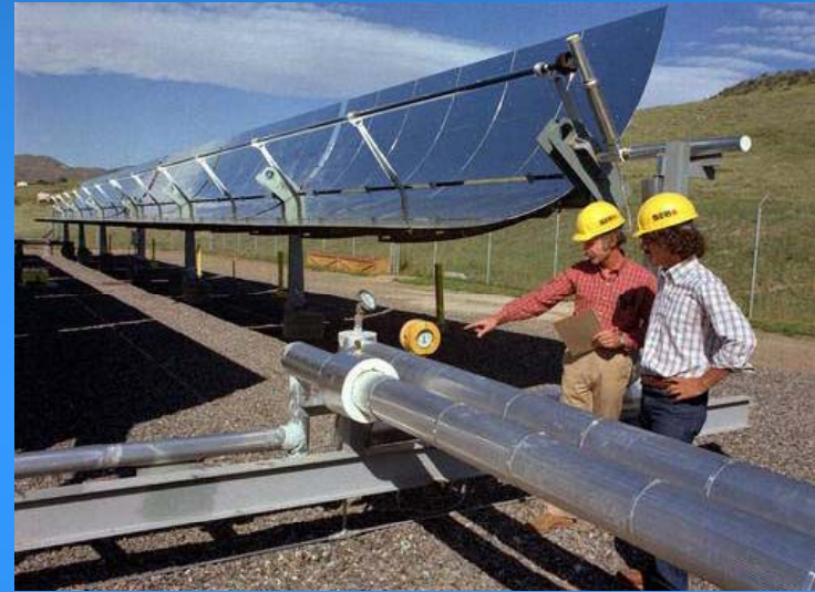
Concentrating Solar Power
