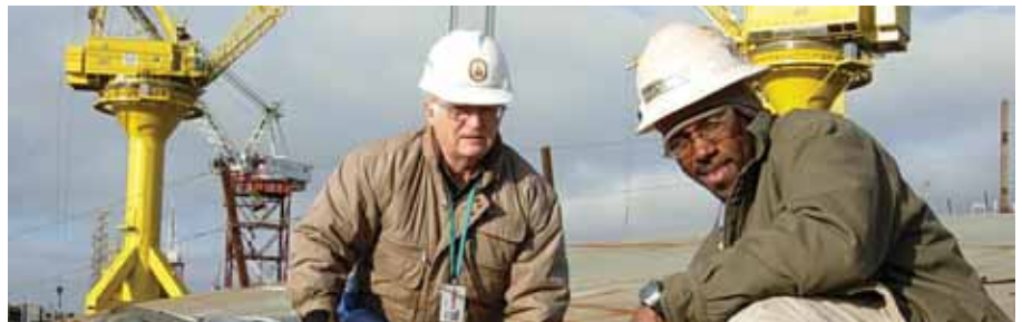
A SUPSHIP Gulf Coast quality assurance specialist inspects a shell plate weld performed by a contractor. U.S. Navy photo
