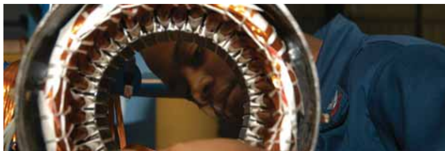
A Sailor rewinds and calibrates a ventilation motor at USS Carl Vinson's (CVN 70) Light Industrial Facility during the ship's refueling and complex overhaul. Photo by MCSA Roderick Barclay
