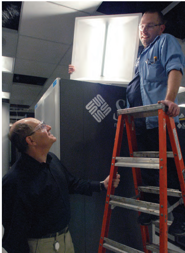
Marvin Kirshenbaum (left, AES-SO) and Robert Brachle (ANL-FMS) with one of the new LED fixtures being installed in the APS computer room. The LEDs help control heat levels in this room in addition to reducing energy consumption.
