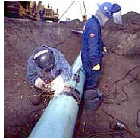
The last weld to the CO 2 pipeline is completed near Estavan, Saskatchewan, in December 1999.
