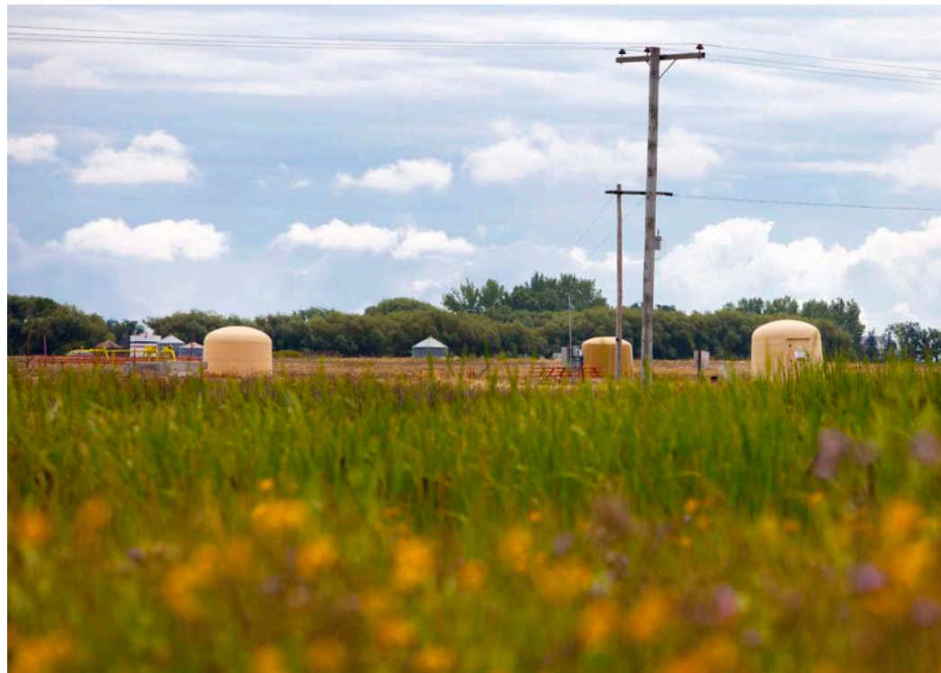
Domes covering CO 2 injector wellheads at the Weyburn CO 2 -EOR project in Saskatchewan, Canada, blend into the landscape. (Courtesy: CCS101)
