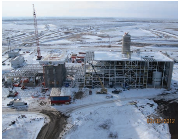
General view of the 1 megatonne/year CO 2 capture plant under construction at the SaskPower Boundary Dam Generating Station near Estevan, Saskatchewan, Canada. (Courtesy: SaskPower)
