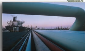
Pipe conveyor oil, Mexico.
