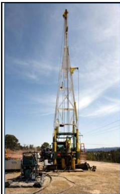
Drilling wells to monitor ground water is an important part of EM work at LANL and other sites.
