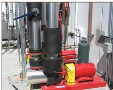
High-efficiency central plant pumps are in place at the Fort Irwin CDC.
