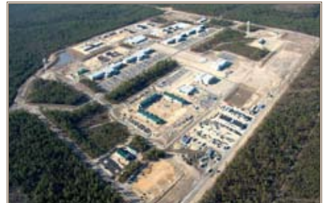
The Corps of Engineers is constructing the new home of the 7th Special Forces Group (Airborne). Photo by Aero Photo
