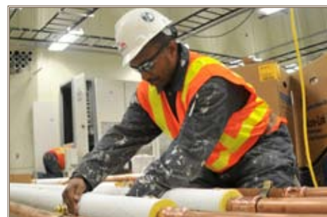
Dwayne Queen, an insulator with TBN-TRA Insulators, installs pipe insulation in the BRAC 133 project site at Mark Center in Alexandria, Va. Photo by Marc Barnes, Belvoir Integration Office, USACE
