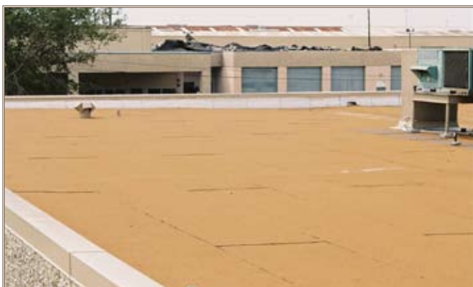
With the roof blown off in background, this roof at the Houston Army Reserve complex, which had been replaced using NRI standards, shows no hurricane damage.
