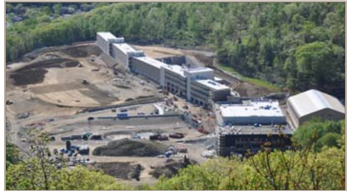
The new U.S. Military Academy Preparatory School is being constructed at West Point by the Army Corps of Engineers' New York District. Photo by Dan Desmet, New York District
