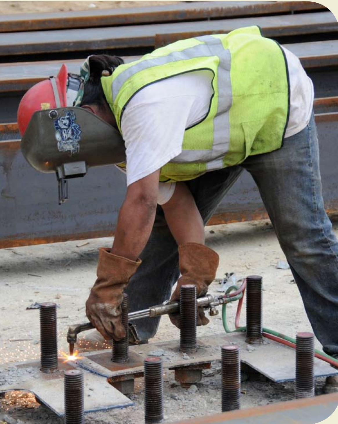
Juan Arango, a steelworker with L.R. Wilson Co., cuts away a template from around anchor bolts at a Base Realignment and Closure project in Alexandria, Va. Photo by Marc Barnes, Belvoir Integration Office, U.S. Army Corps of Engineers. Page 21
