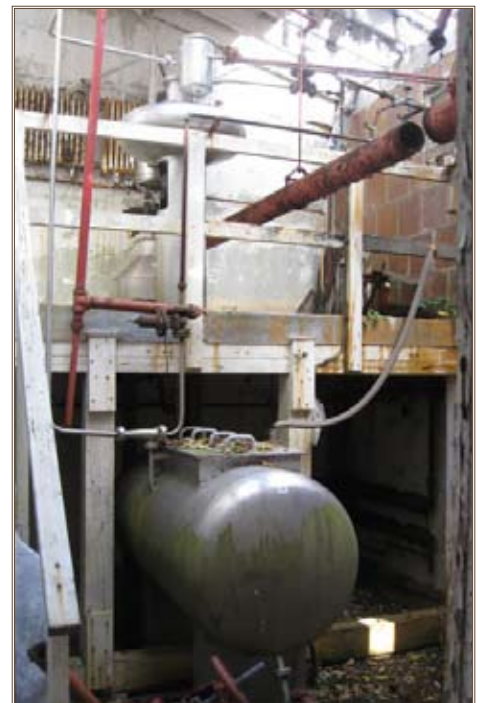
Equipment in the former High Explosive Nitration Building must be decontaminated as part of the removal process for unsafe structures at Picatinny Arsenal. Photos by James B. Smith
