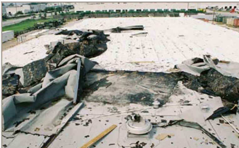
This Army Reserve complex roof in Houston, which had not been replaced under the NRI, shows considerable damage from Hurricane Ike in 2008. Photos by Bud Lewis
