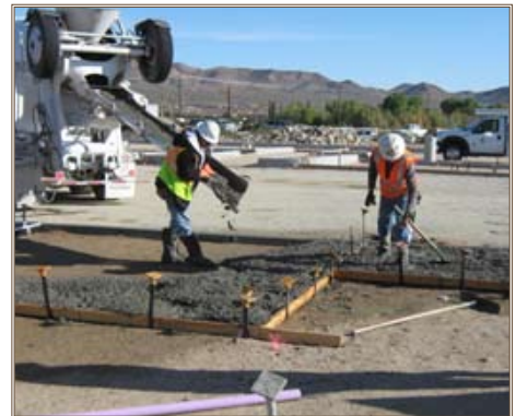
Workers place concrete at the entrance to the Fort Irwin CDC. Photos by Paula M. Dolliver-Marshall, U.S. Army Corps of Engineers
