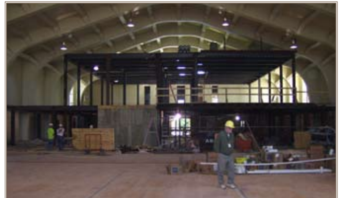
A new structure is built inside the drill hall of the Urbana, Ill., armory. Photos by Kyle Blumberg, Illinois Department of Military Affairs
