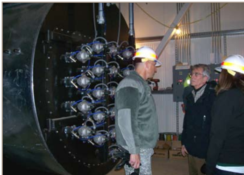
New York District Commander Col. John R. Boulé discusses the project with district employees Robert Philbrick and Lucia Gamba in front of one of several newly constructed exhaust gas boilers the Corps built at Thule Air Base.
