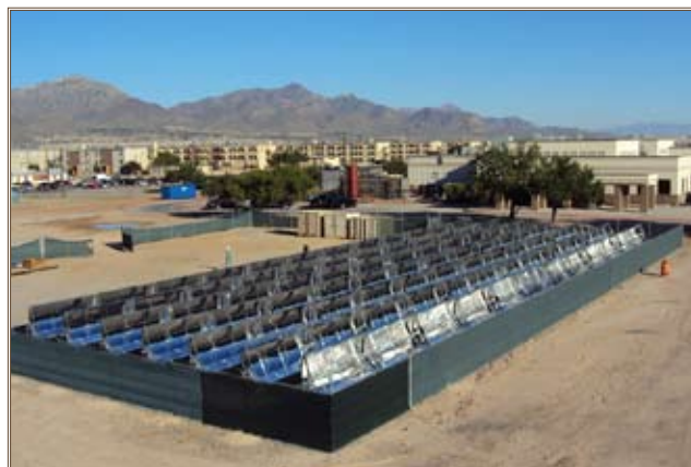
A parabolic hot water array provides preheated domestic hot water for the Stafford Dining Hall at Fort Bliss as part of an ESPC project. By producing and consuming renewable energy on-site, Fort Bliss also receives double credit toward Energy Policy Act 2005 goals. Photo courtesy of Jon Crowell, JCI
