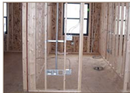
Improper "construction" is discovered inside a purchased RLB.
