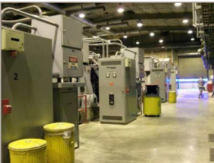
The generators in the M-Plant deliver power for heating and hot water at Thule Air Base. Photos by JoAnne Castagna
