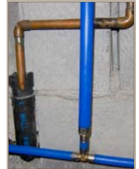
PEX piping is installed in conjunction with copper piping at Fort Campbell. Photo by Louis Bartels
