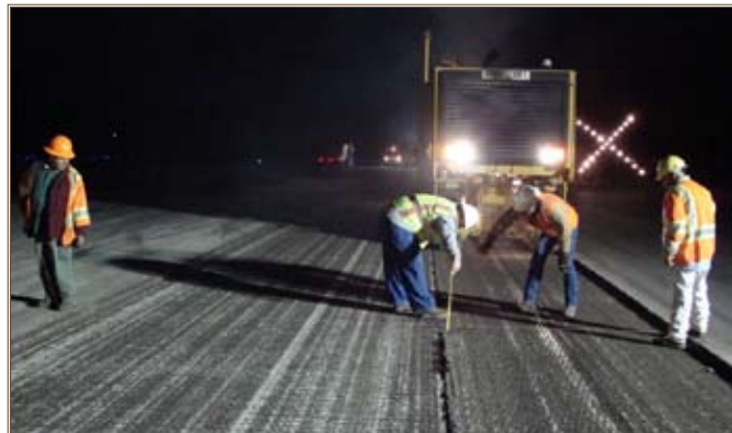
Workers measure depth after milling operations during rehabilitation of the joint-use runway at Fort Hood. Photos by Patrick Spilman, Central Texas Area Office
