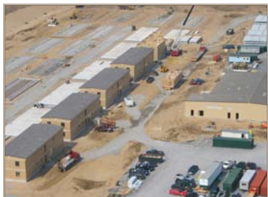
RLBs are improperly "constructed" on site. Photos courtesy of Barry Bartley
