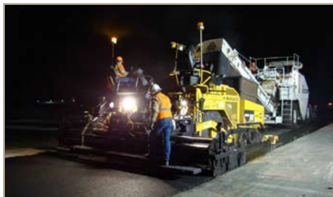
Runway paving is done at night, so that flight operations can continue during the day.
