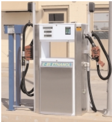
The newly installed E-85 dispenser is constructed of non-corrosive materials required to handle ethanol.
