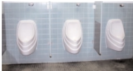
Installations that use waterless urinals to replace traditional flush fixtures are conserving millions of gallons of water each year, in addition to avoiding repair costs.
