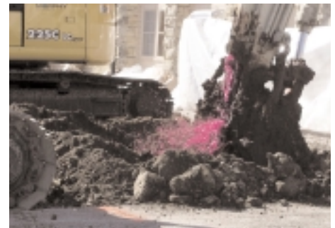
A machine injects liquid potassium permanganate into a cleanup site on Fort Riley, Kansas.
