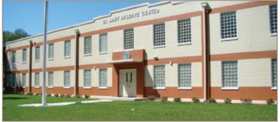
The Gainesville, Fla., Army Reserve Center sports a fresh, clean look following a $5.1 million renovation. Photos by Lt. Col. Brian Griffin, Office of the Assistant Chief of Staff for Installation Management
