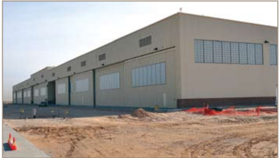
The aviation support brigade hangar is under construction on Biggs Army Airfield. Photos by Virginia Reza
