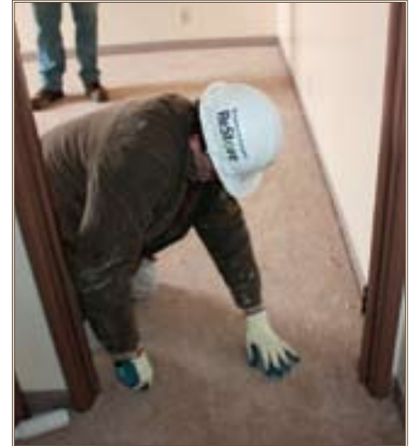
ReStore worker James Stowe prepares carpet for removal from a Fort Riley home that is scheduled for demolition. Photo by Stephanie Hoff
