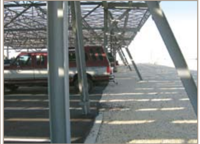
Web steel joists and joist girders will support the steel carport structures above the parking lot pavements.
