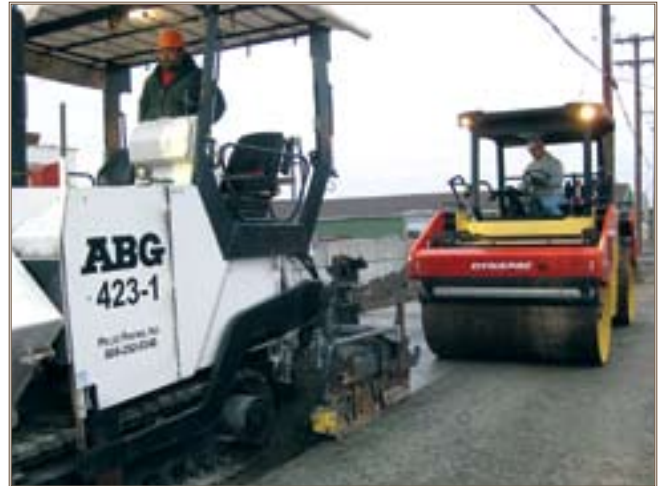
Contractors place and compact concrete using cold RCC technology during a field demonstration at Fort Drum March 31. Photo by L. Barna, CRREL
