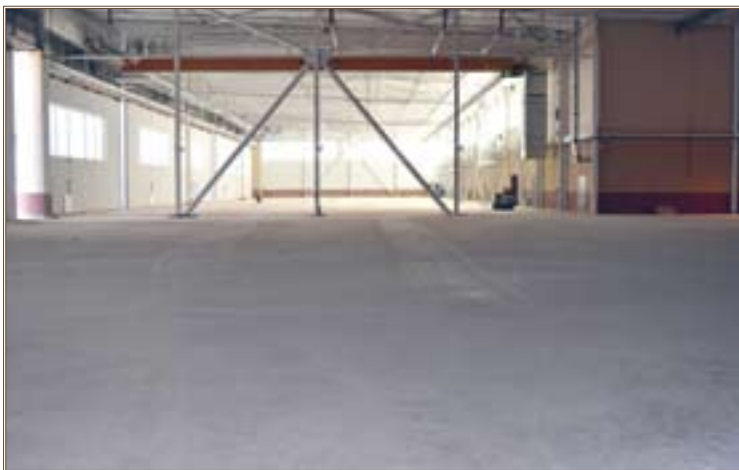
This aviation support hangar will house CH-47 Chinook aircraft in the fall of 2011.
