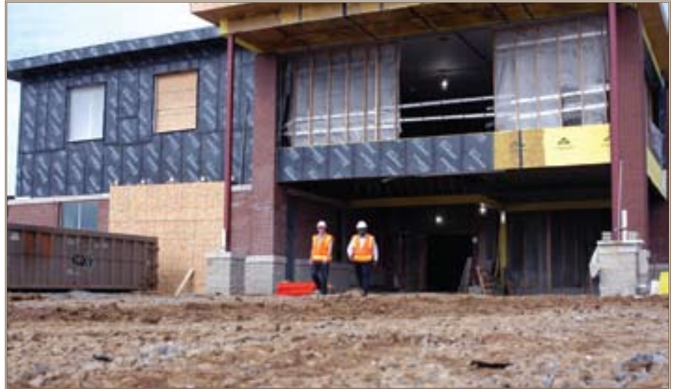
Two Louisville District U.S. Army Corps of Engineers employees walk out of the New Fort Knox High School during construction. The school was completed in May. Photos by John Neville
