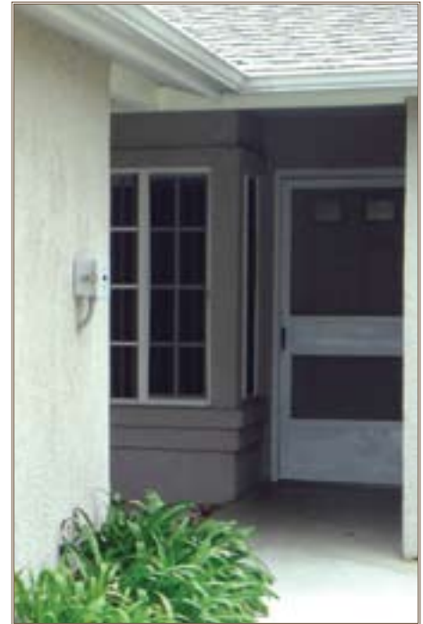
The unobtrusive outdoor meter in a NEMA 4 weatherproof enclosure is installed near the entry to a typical Camp Pendleton housing unit, allowing fast, accessible utility data collection. Photo courtesy of Hondo Electric
