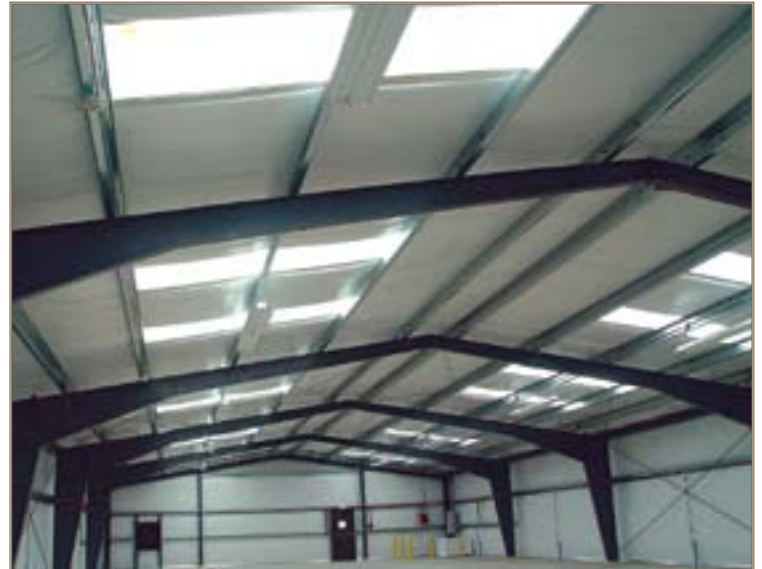
Skylights in the roof of Fort Irwin's net-zero energy building provide lighting during daylight hours. Photos by Hossam Kassab
