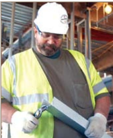
A contractor cuts metal at the site of the new Fort Knox High School.
