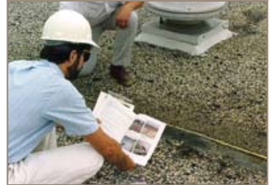
Workers perform ROOFER distress survey with visual guide book. Graphic and photo courtesy of the Engineer Research and Development Center
