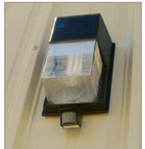
Exterior lighting fixtures have light-sensitive photocells that turn the lights on only when it is dark outside.
