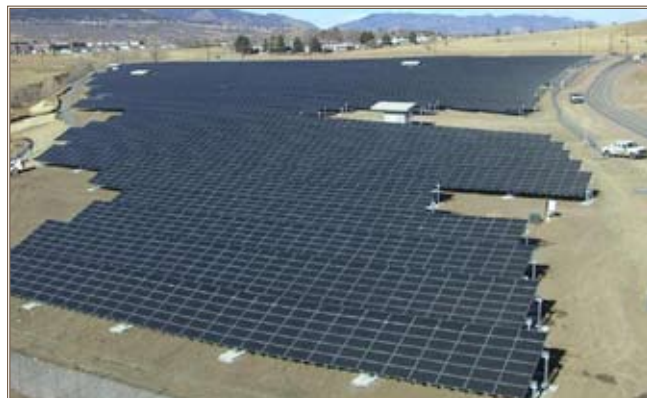
Fort Carson, Colo.,'s solar array generates renewable energy. Photo courtesy of Fort Carson
