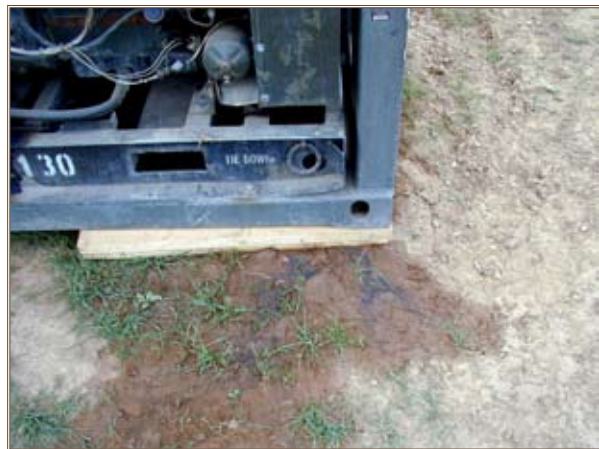
An SPCC requirement is to periodically inspect oil-using equipment, like this generator, for possible wear, leaks or seepage. Photo by Dana Finney
