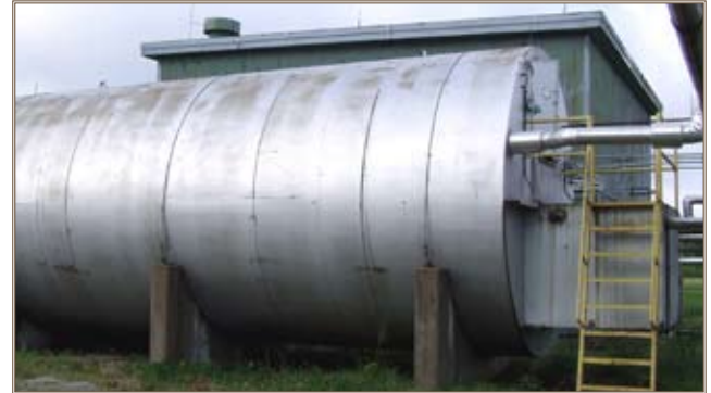
The recirculation system at IAAAP includes several holding tanks with secondary containment, pumps and an alarm system. Photo by Keith Miller
