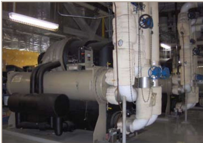
A chiller unit at Madigan Army Medical Center uses nonpotable water that is later reused for irrigation. Photos by Bob Cody, Madigan Army Medical Center
