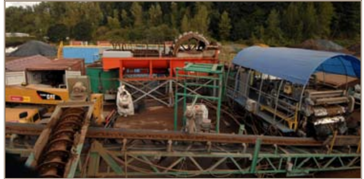
This equipment uses a multi-stage process to treat contaminated soil from the Camp Withycombe cleanup. Photo courtesy of the Oregon Military Department Public Affairs Office
