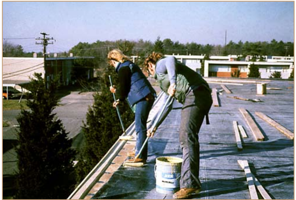
The National Roofing Initiative requires a 20-year manufacturer’s guarantee for roofs. Photo courtesy of the U.S. Army Engineer Research and Development Center
