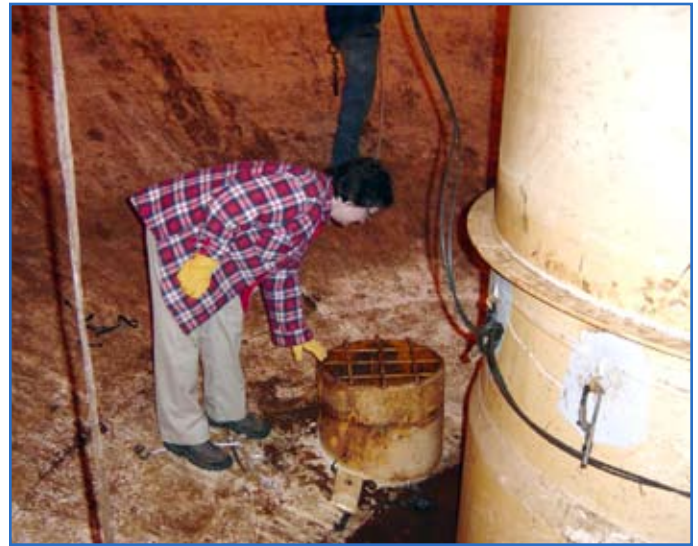
Vicki Van Blaricum, who managed the Fort Drum project, checks on the progress of work inside the bowl of the tank during the installation of the ice-free corrosion prevention system. Photo by John Field
