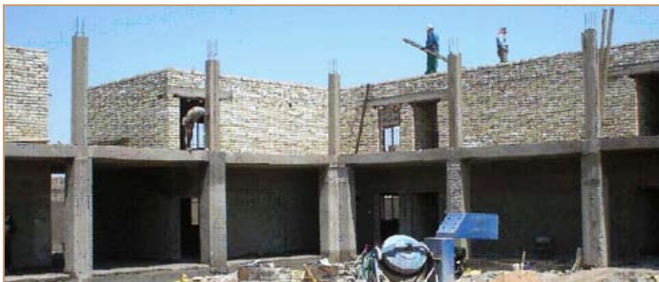
Ghassem Khosrownia worked with Iraqi contractors on this addition to the Taji Girls’ School, a new 1,350-square-meter, two-story structure that will benefit 700 high school students. Photo by Norris Jones
