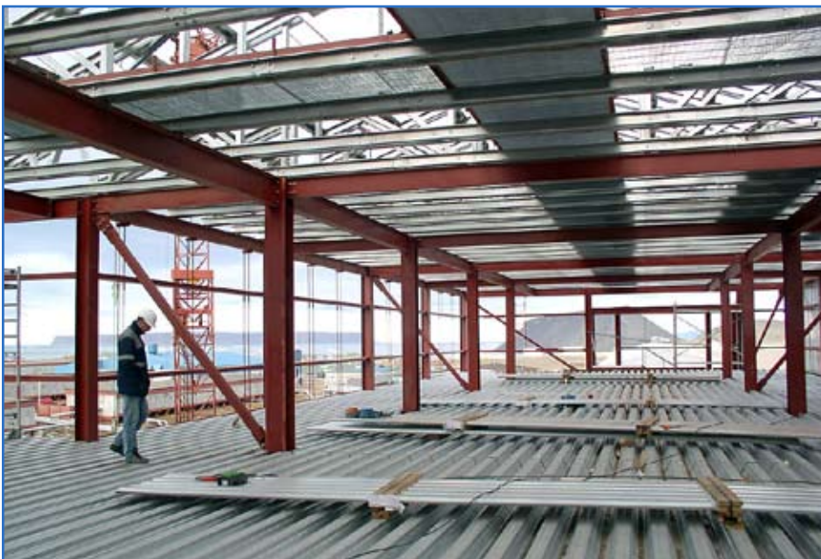
Contractors inspect installation of flooring system metal decking. Photo by Sterrett Daniels, U.S. Army Corps of Engineers, New York District
