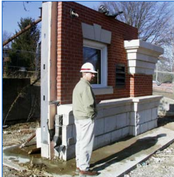
David Manka, project manager for the Lewis and Clark Classroom Facility at Fort Leavenworth, Kan., explains details of the building's structure using a section of sample wall built by the contractor. The facility's brick exterior masks its structural steel, giving it architecture similar to historic structures at Fort Leavenworth. Photo by Eric Cramer
