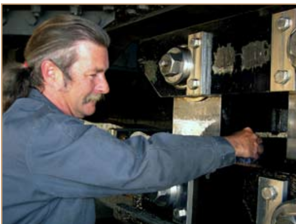
Rick Simpson, Government Bridge groundsperson, wipes off dirt from the swing span lift mechanism. Photo by Valerie Buckingham
