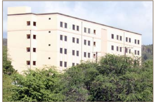
The exterior work is done on Favreau Hall at Fort Shafter, and crews are focusing on the interior work needed to be ready for Soldier occupation later this year. Photo by Lacey Justinger
