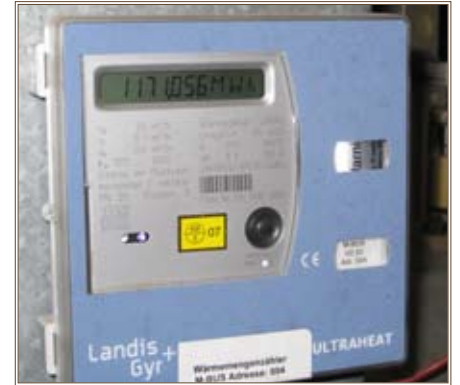
Meters installed on reimbursable tenant buildings ensure that tenants are accurately billed for their utility use. Photo by Gary Harper, project engineer, Huntsville Center
