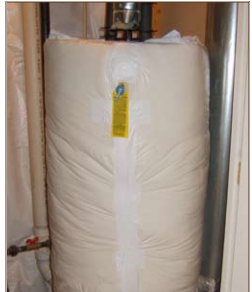
Adding insulation to water heater tanks reduces standby heat losses. Photos by Matthew D. Conlan
